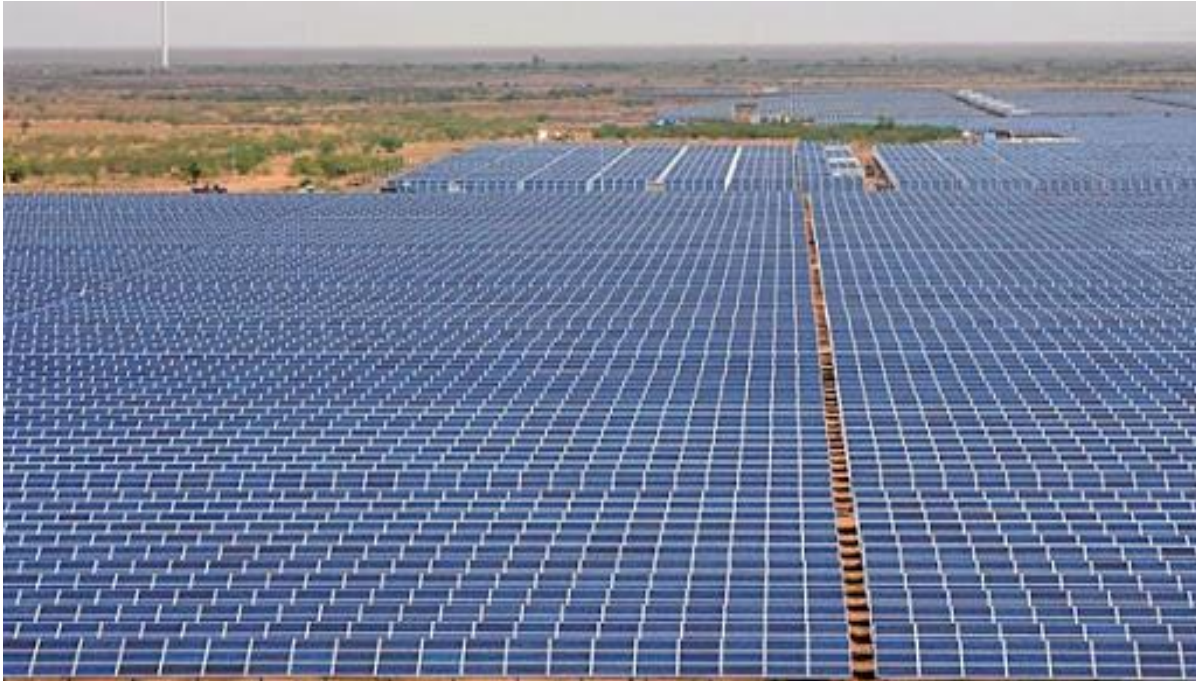
Fig 2.2: Indian Biggest Solar Power Plant
