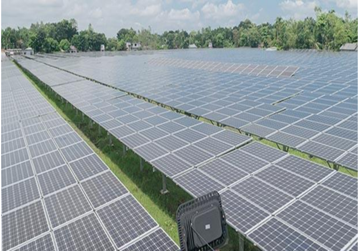
Fig 2.3: Bangladesh Largest Solar Power Plant
