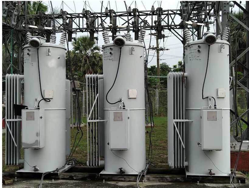
Fig-4.7: Voltage Regulator
