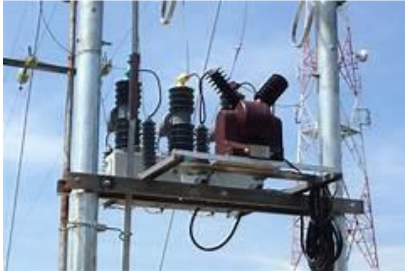
Fig-4.4: Automatic Circuit Recloser
