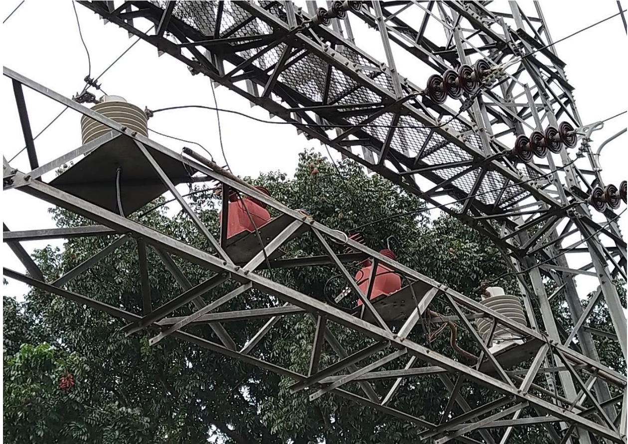
Fig-4.5: Current Transformer (CT) & Power Transformer (PT)
