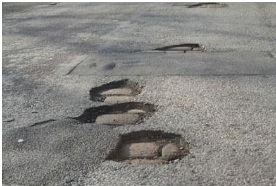
Figure 2.2.1: Pothole image sample.
