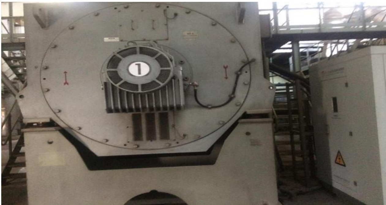
Figure 3.13 Generator at Santahar power Plant
