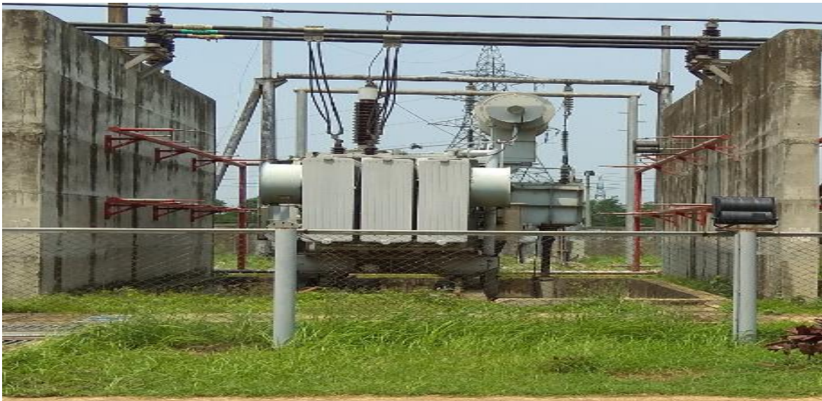
Figure 4.4 Power Transformer-2 of Santahar
