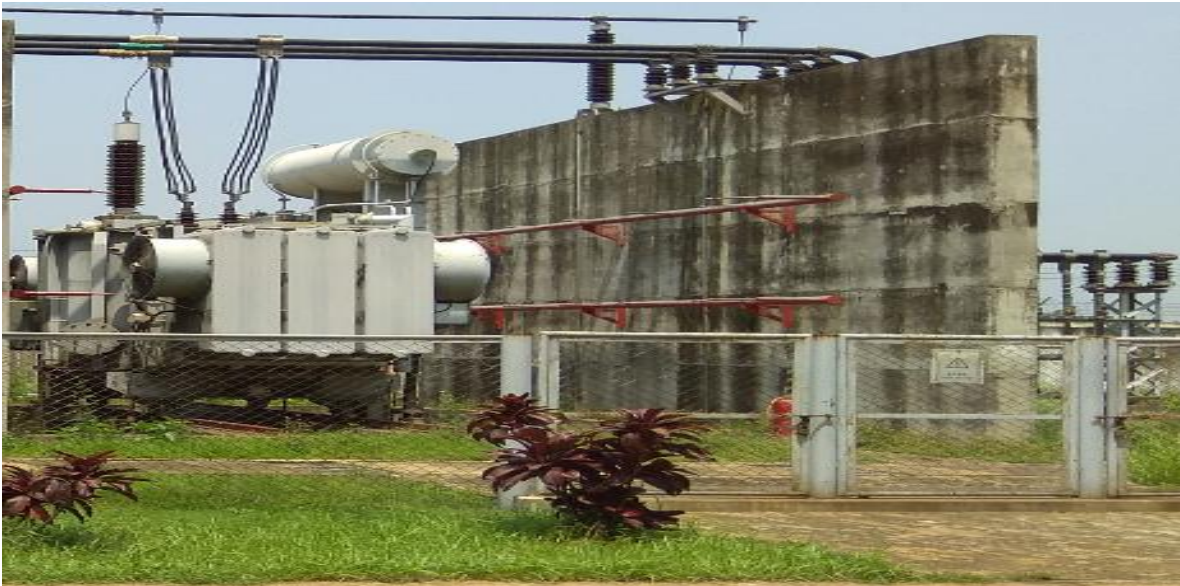
Figure 4.3 Power Transformer-1 of Santahar
