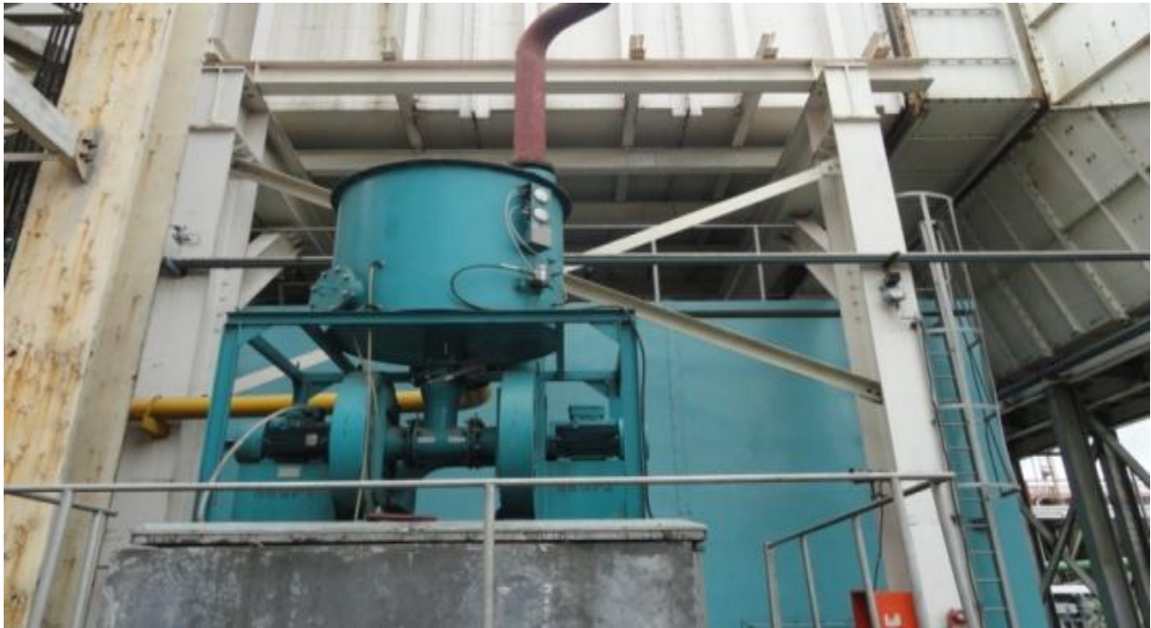
Figure 4.6: Moist Eliminator Pump of Santahar
