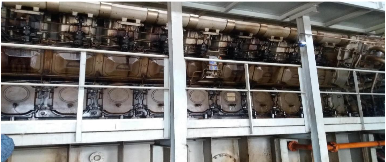
Figure 3.12 MAN18V32/40 Diesel engine at Santahar
