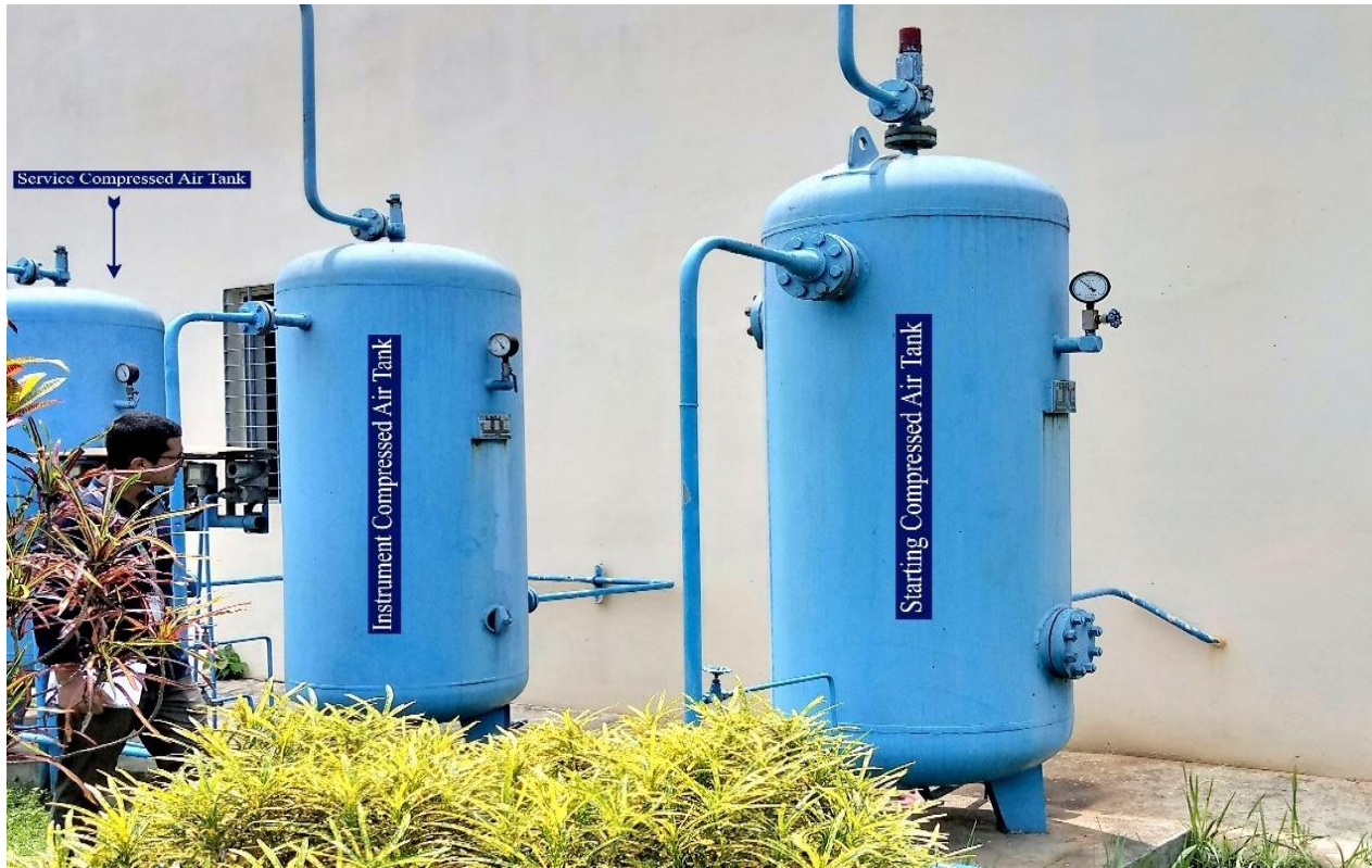
Figure 3.5 Compressed Air Tanks
