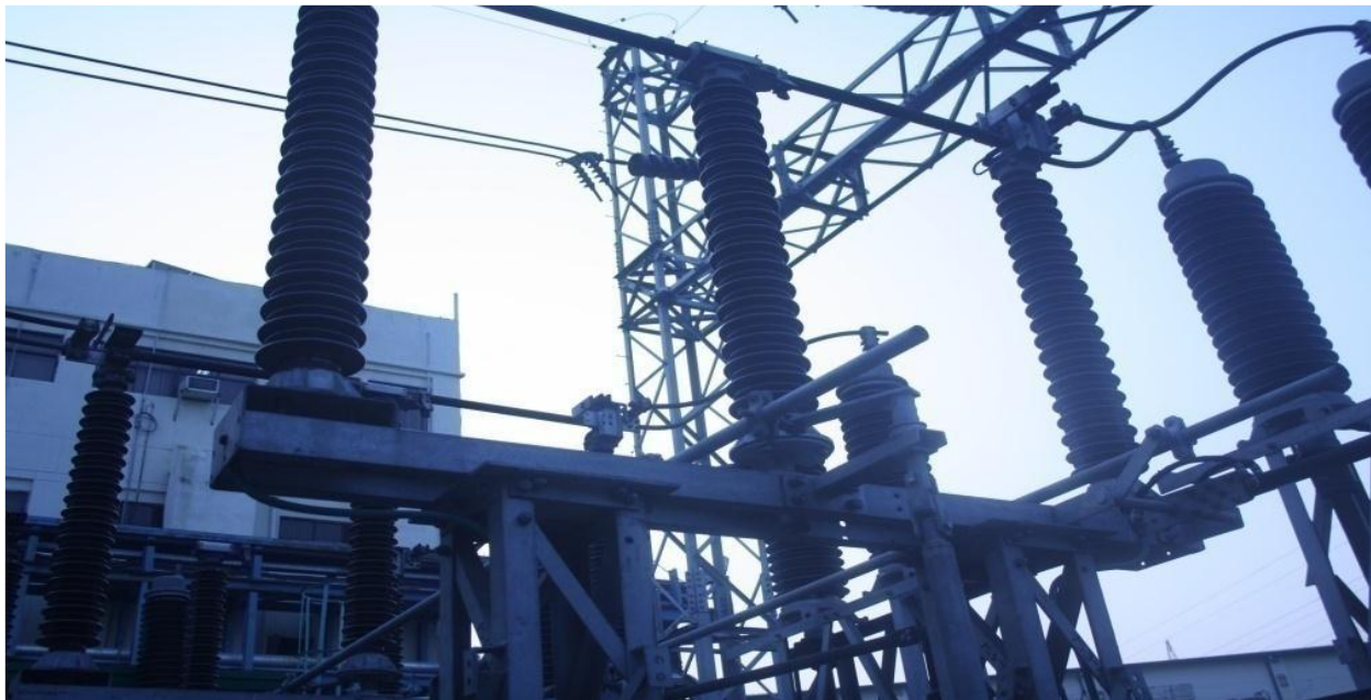
Figure 4.7: Different types of Insulators used in Santahar substation
