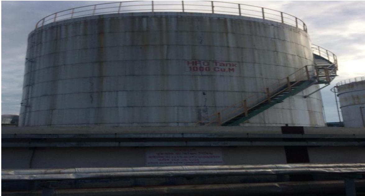
Figure 3.7 HFO tank at Santahar power plant
