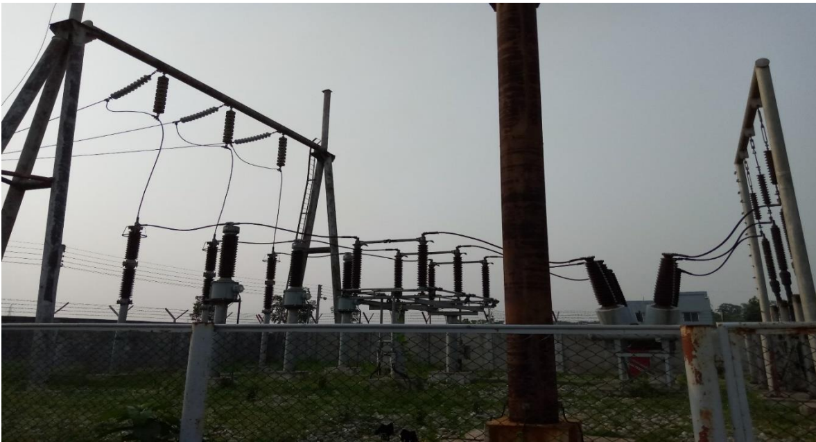
Figure 4.2 Substation of Santahar
