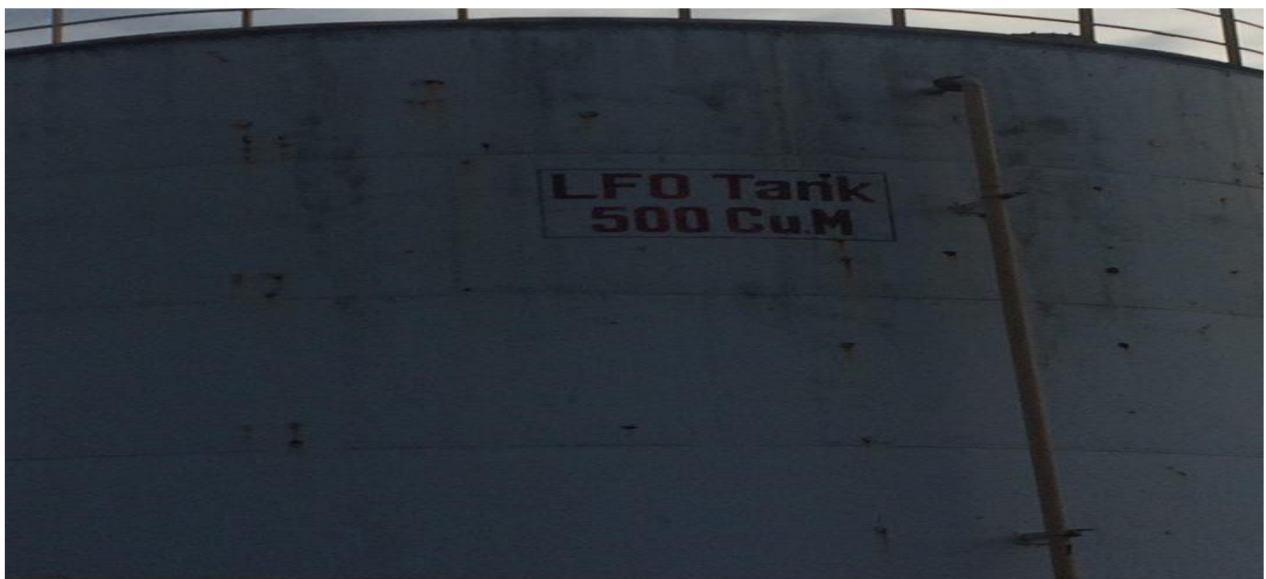
Figure 3.8 LFO tank at Santahar power plant
