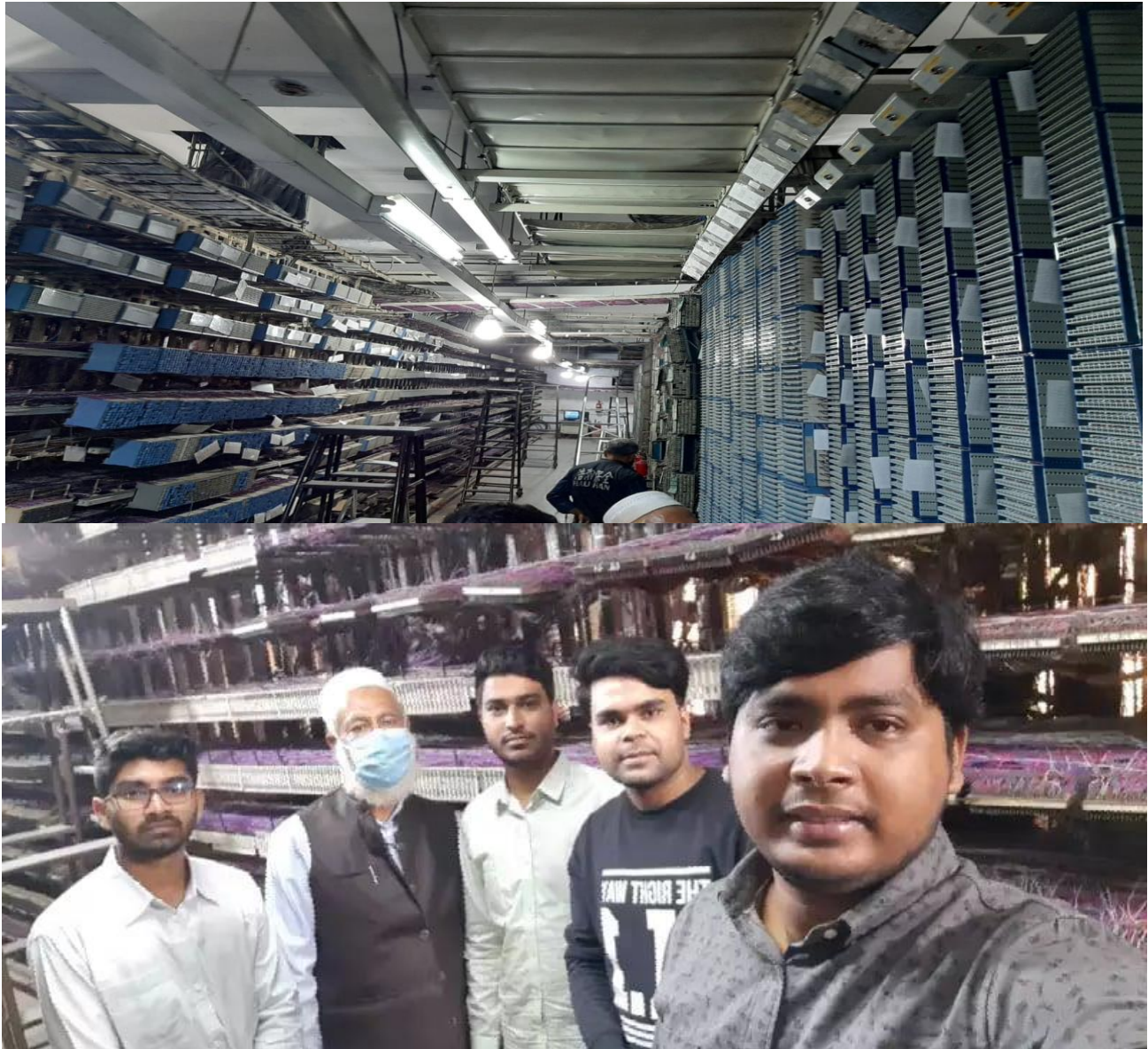
Figure 3.3: Modern Main Distribution Frame (MDF)
