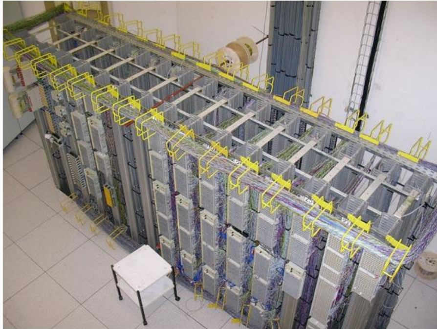
Figure 3.7 Modern main distribution frame
