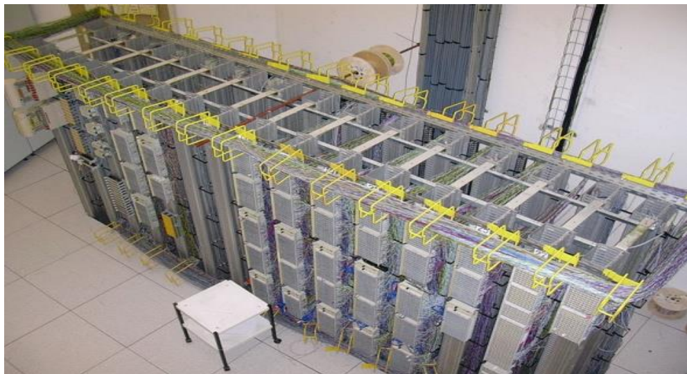
Fig: 3.2 Main Distribution Frame
