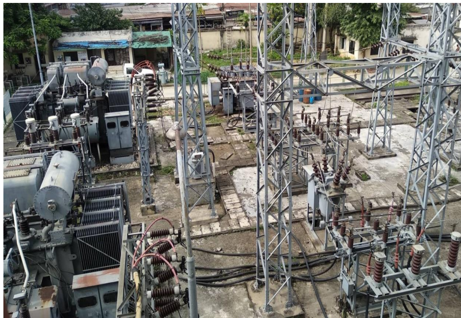
Figure 4.2: Madertake is a 132/33/11 KV substation
