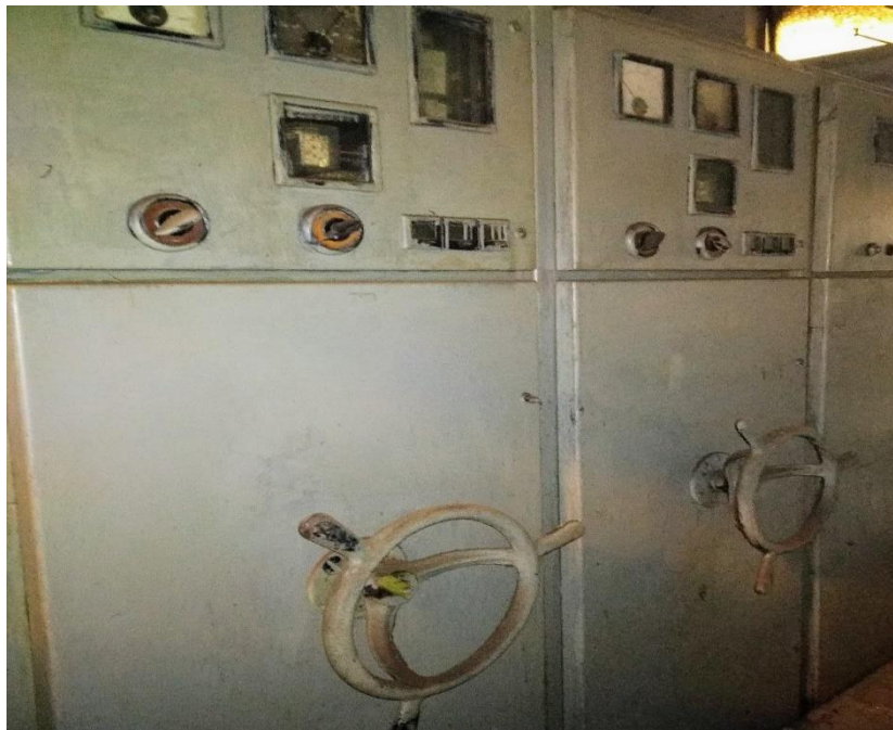
Fig 4.2 Oil circuit breaker
