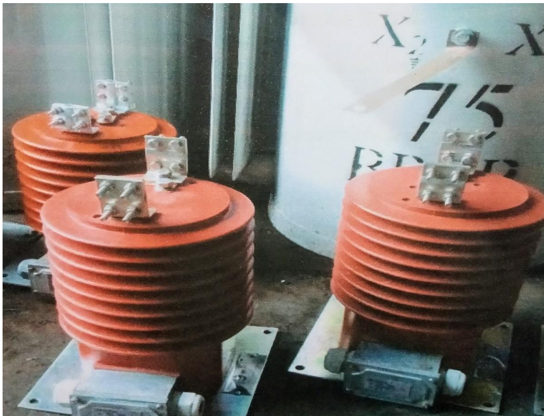
Fig 3.2 Current Transformer (CT)
