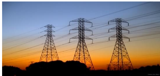
Figure 2.8: Overhead Transmission Line
