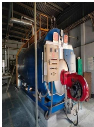
Fig: 4.2 Boiler machine
