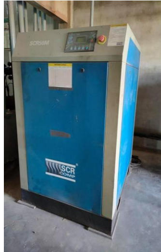
Fig: 4.1 Air compressor machine
