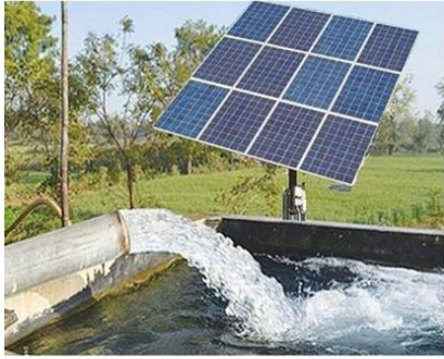
Fig.2.17: Solar water pump
