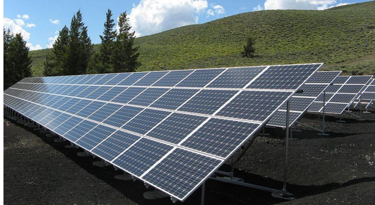
Fig.2.15: Photovoltaic solar panel
