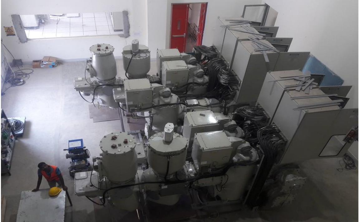
Figure: 2.3: SF6 circuit breaker
