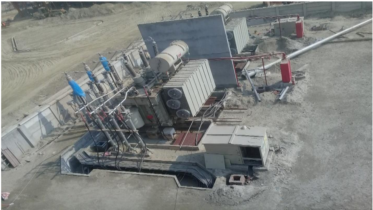
Figure: 2.1: 132/33 KVA sub-station
