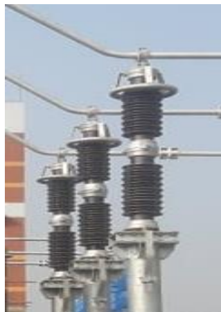
Figure: 2.10 Lightning arrester.
