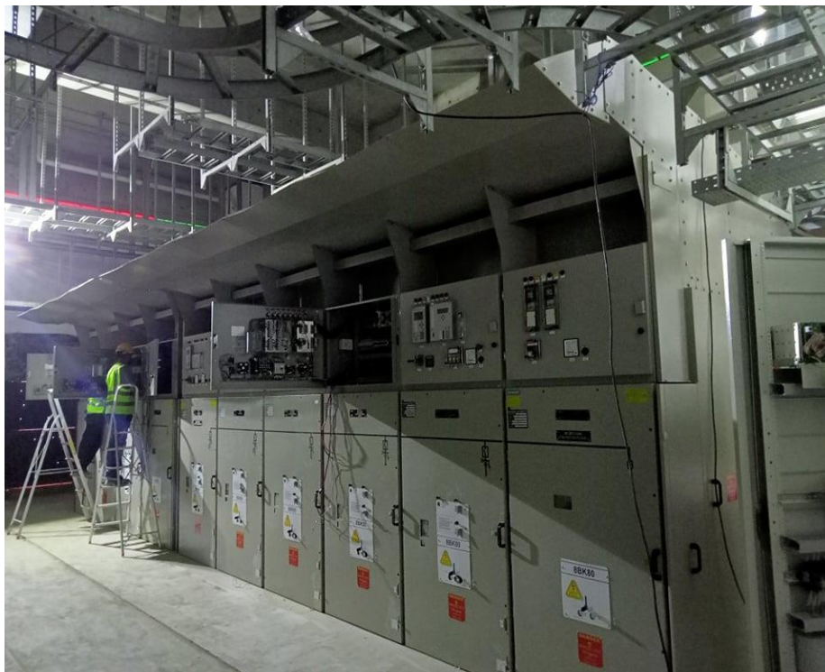
Figure: 2.13: 33KV Switchgear Panels
