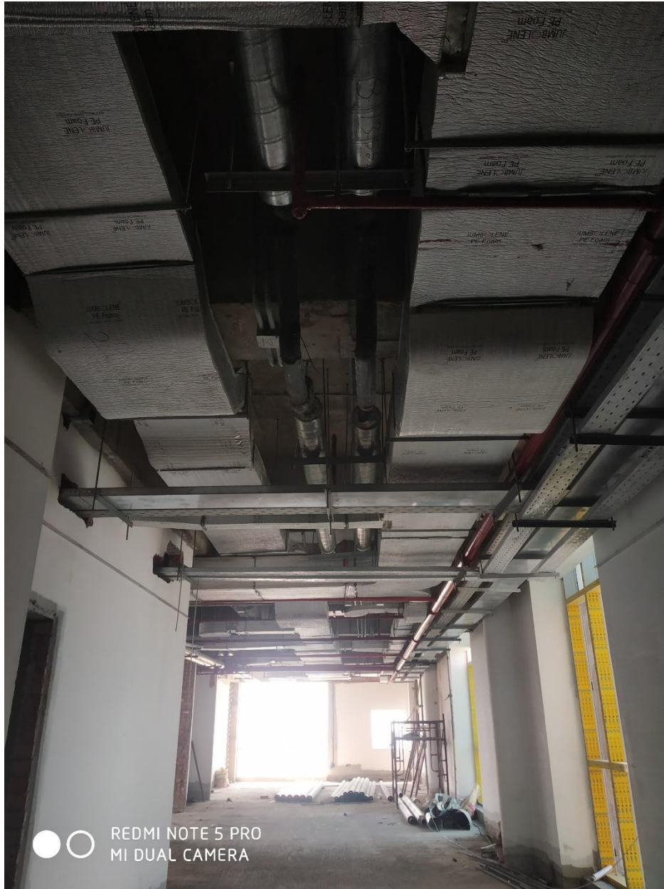
Figure: 4.3: Channel cable Tray
