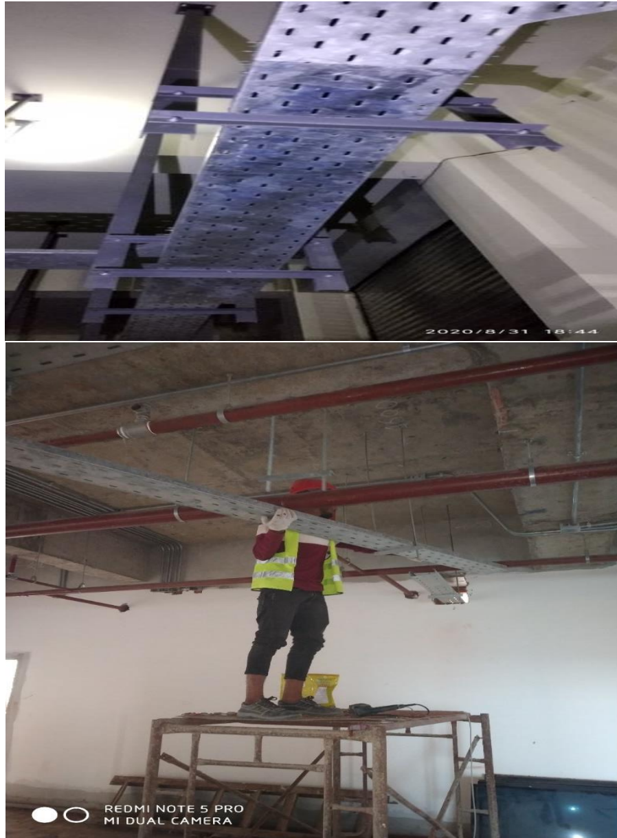
Figure: 4.2: Perforated Cable Tray
