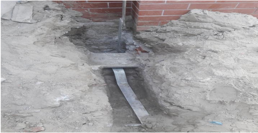
Figure: 2.18: GI flat bar earthing
