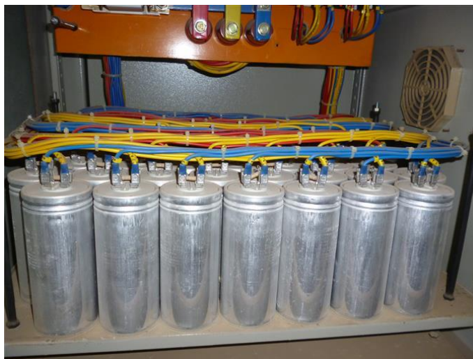
Figure: 2.12: Capacitor Bank
