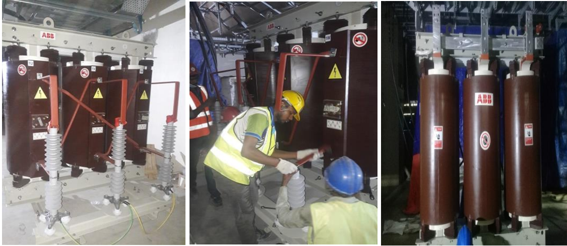
Figure: 2.15: Dry Type Transformer
