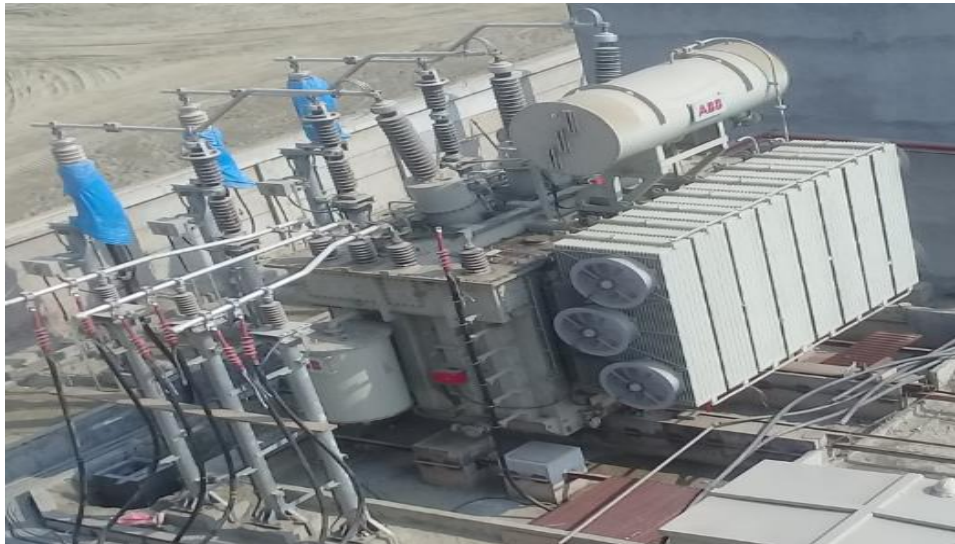
Figure: 2.5: Power Transformer
