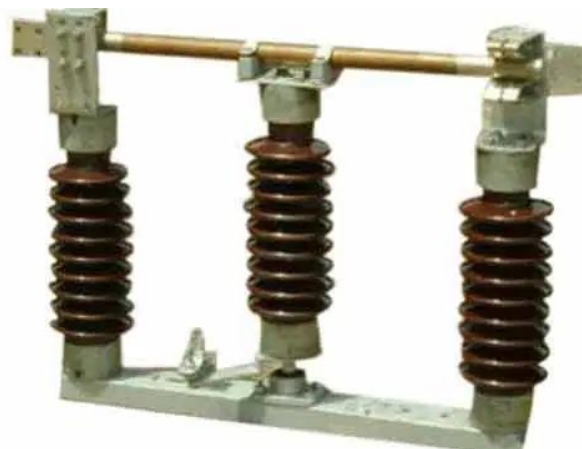
Figure: 2.4: Double break type isolator
