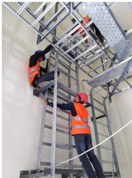
Figure: 4.1: Ladder cable tray
