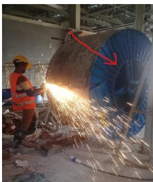
Cable puller and tensioner
