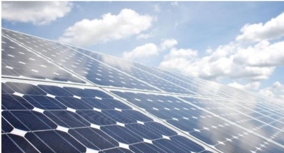
Power plant - Photovoltaic
