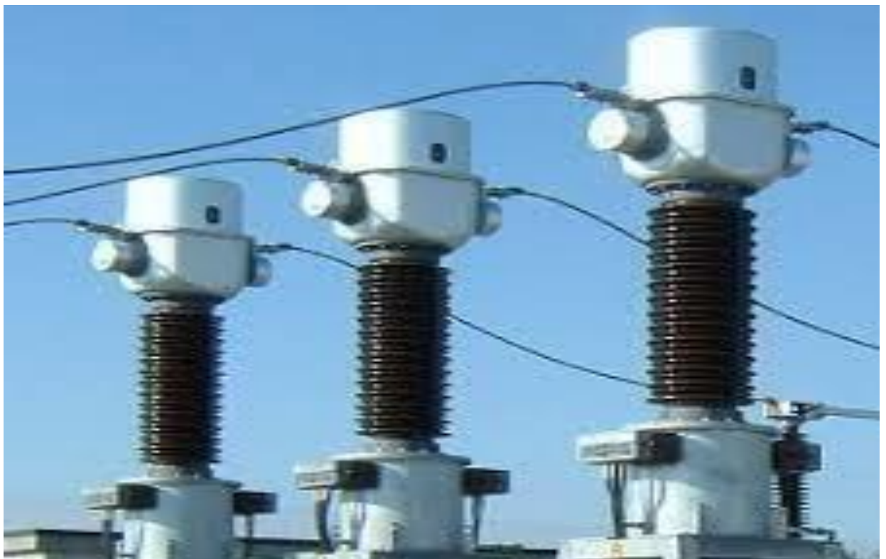
Fig. 3.6 Potential Transformer (PT)
