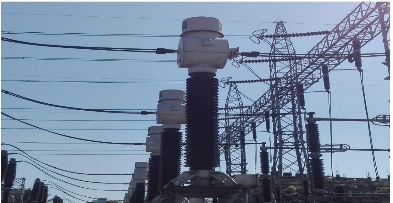
Fig. 3.4 Current Transformer (CT)
