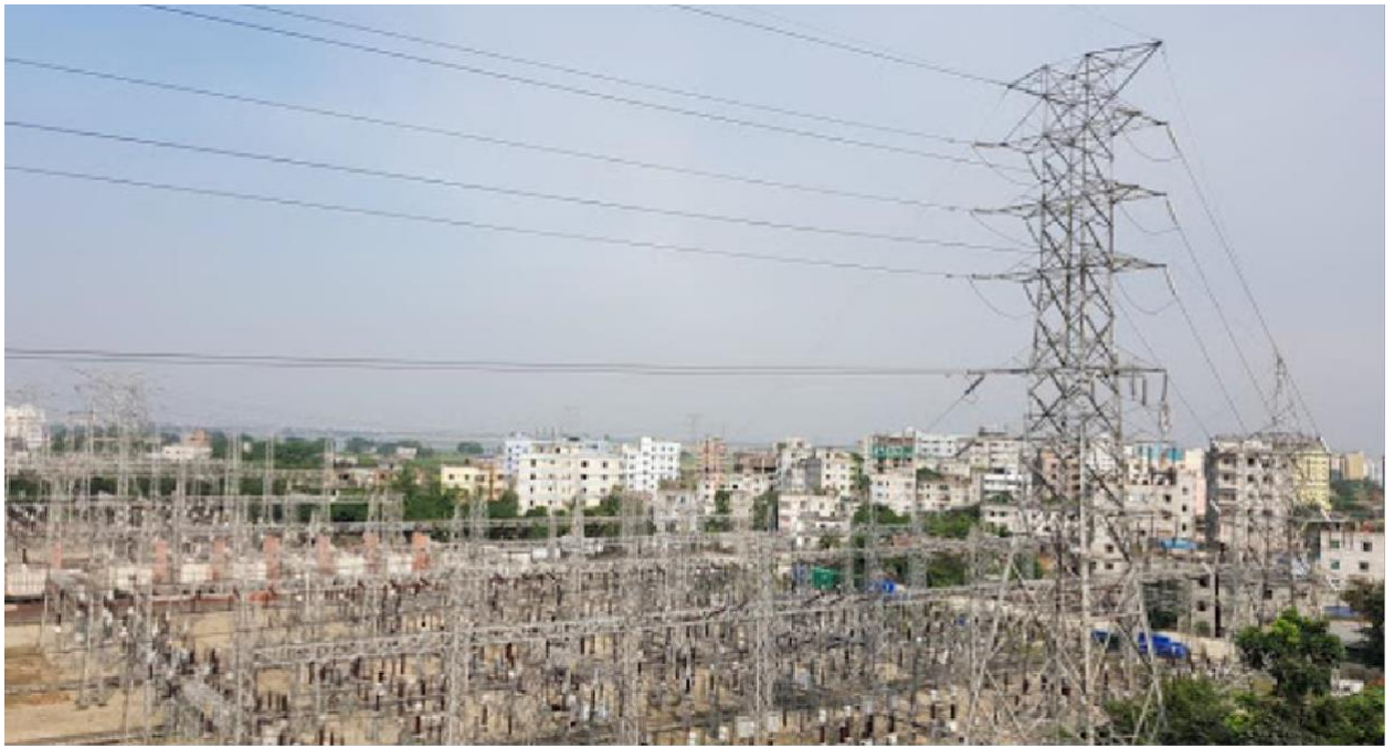
Fig. 2.1 Rajendrapur 132/33 KV grid substation
