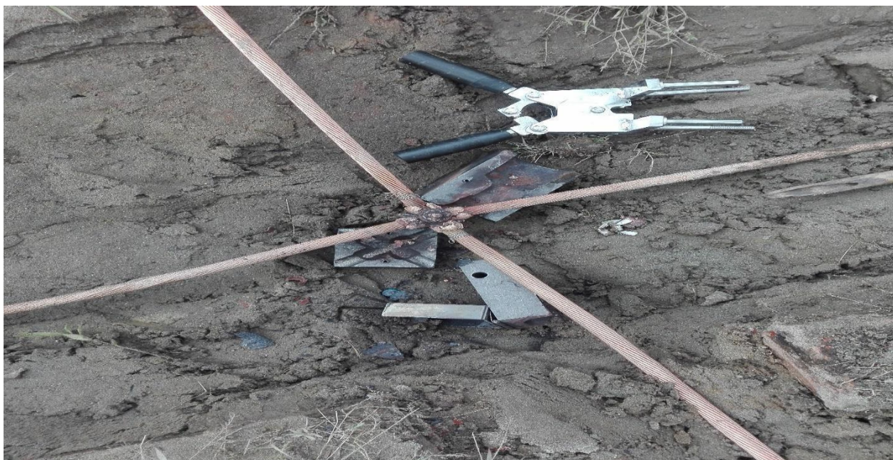
Fig. 4.1 Earthing of Rajendrapur 132/33 KV grid substation
