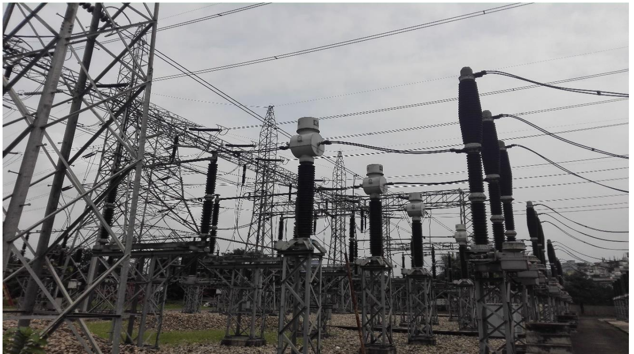
Fig. 2.2 Elements of Rajendrapur 132/33 KV grid substation
