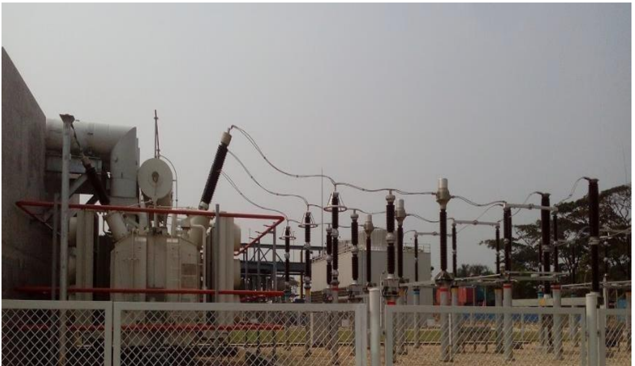
Fig. 2.3 Rajendrapur 132 KV Gas Insulated Substation
