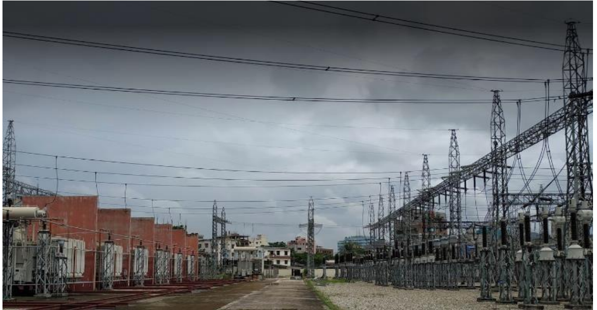
Fig. 3.1 Rajendrapur 132/33 KV grid substation
