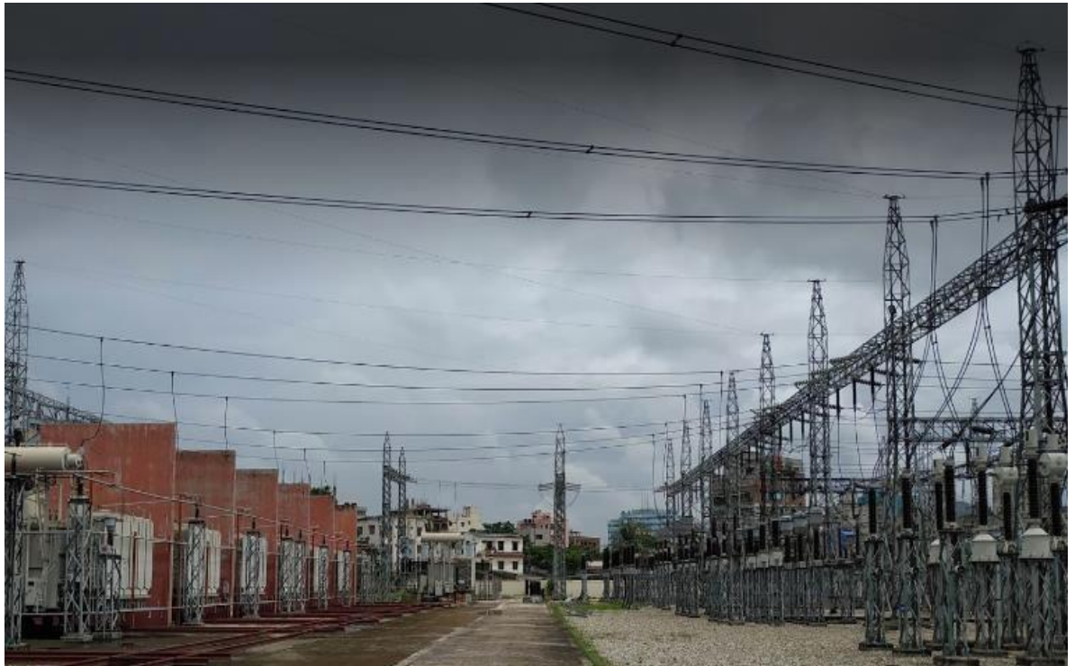
Fig. 2.4 Rajendrapur 132/33 KV grid substation
