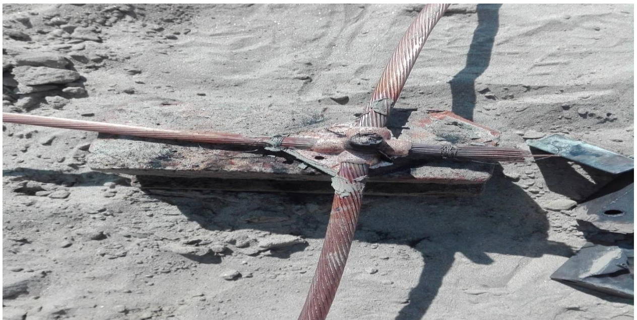
Fig. 4.4 Joint of sub mass with main mass in Rajendrapur 132/33 KV grid substation
