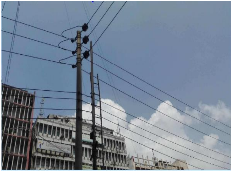
Figure 3.9.1 11 KV/ LT Line with Jumper
