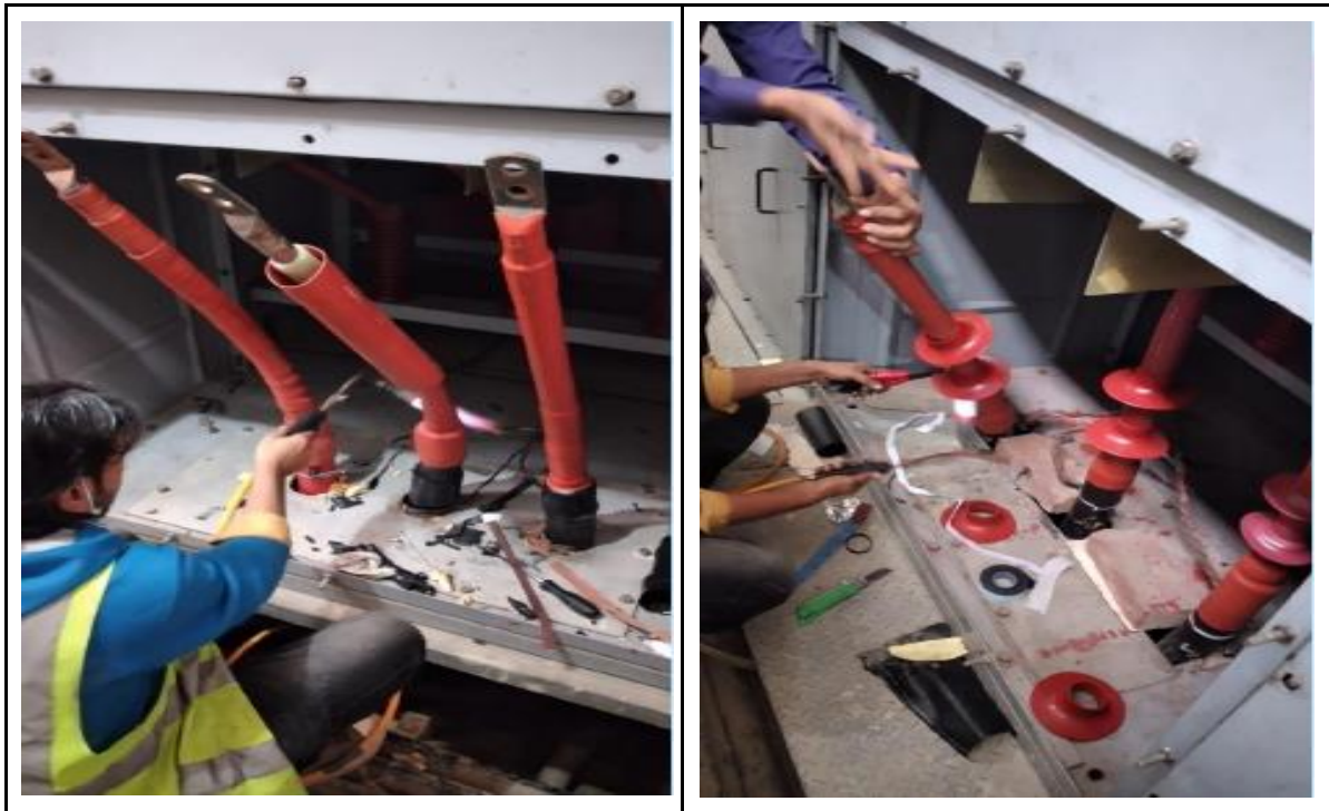
Figure 3.11.1 Cable Connection in Substation Breaker
