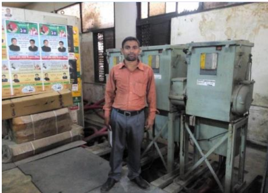
Figure 3.6.1 11 KV RMU ( Ring Main Unit )
