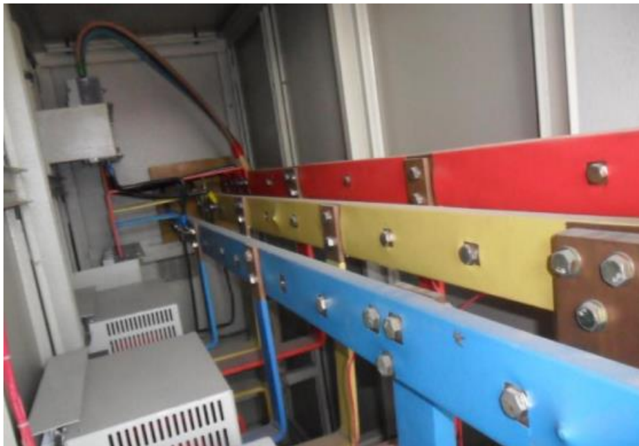
Figure 3.4.1 11 KV Bus Bar
