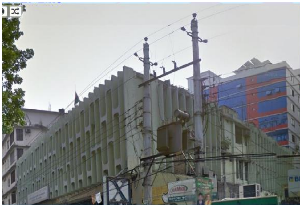
Figure 3.8.1 11 KV/ LT Line
