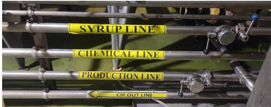
Fig 11: Raw Materials Production Line
