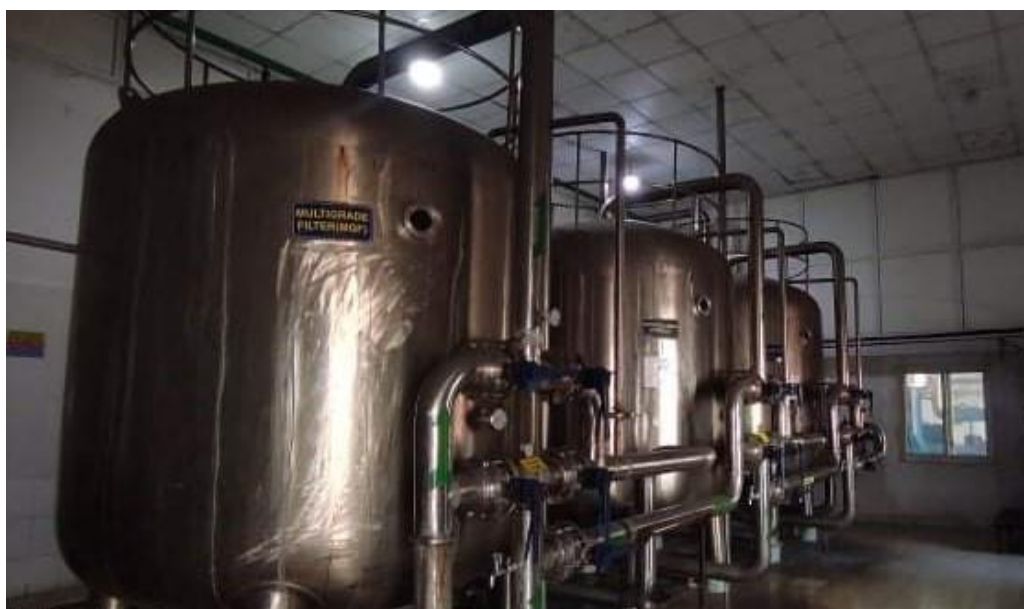
Fig 2: Water Treatment Plant (WTP)
