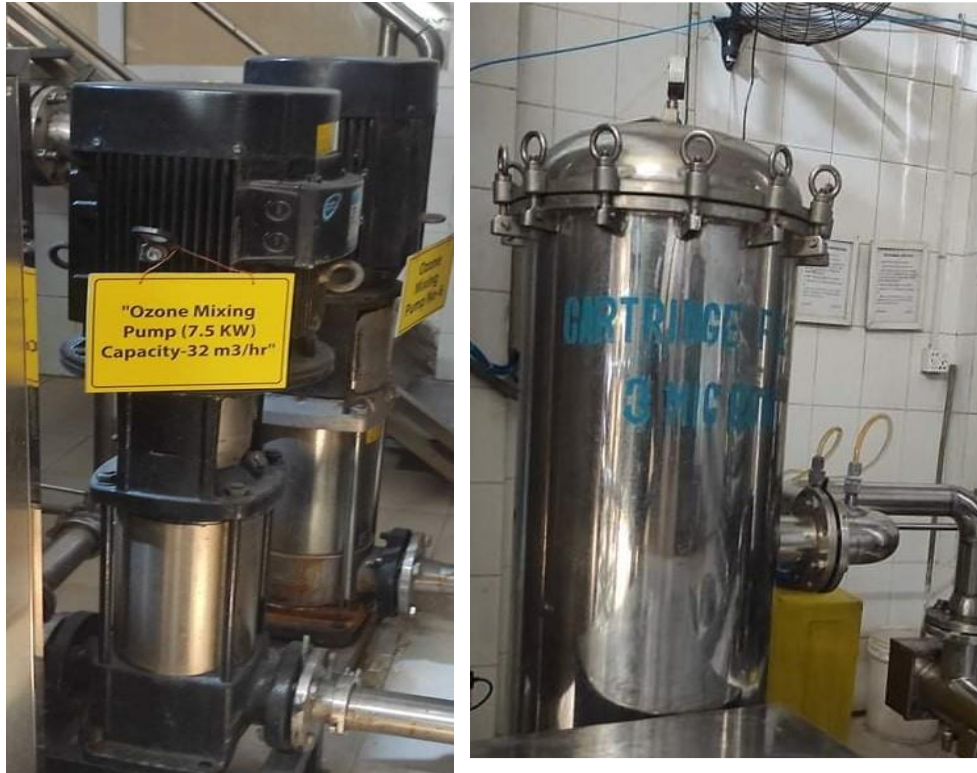
Fig 4: Ozone mixing pump & Cartridge filter
