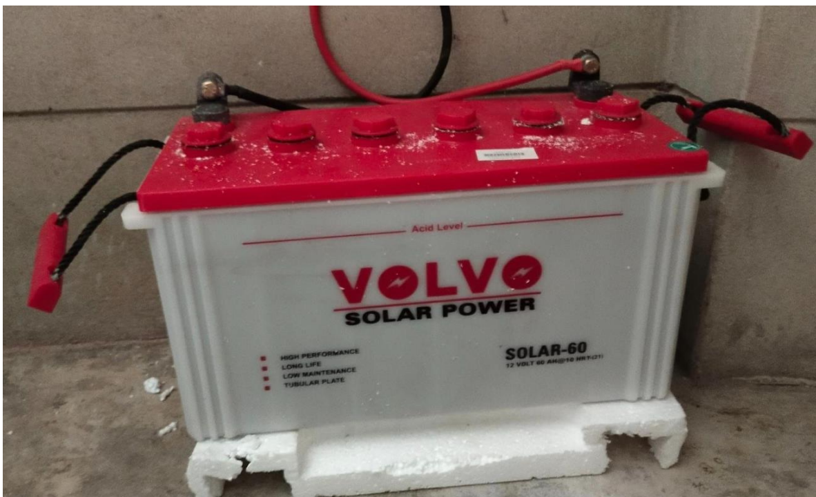
Figure 4.13: Batteries of the solar system
