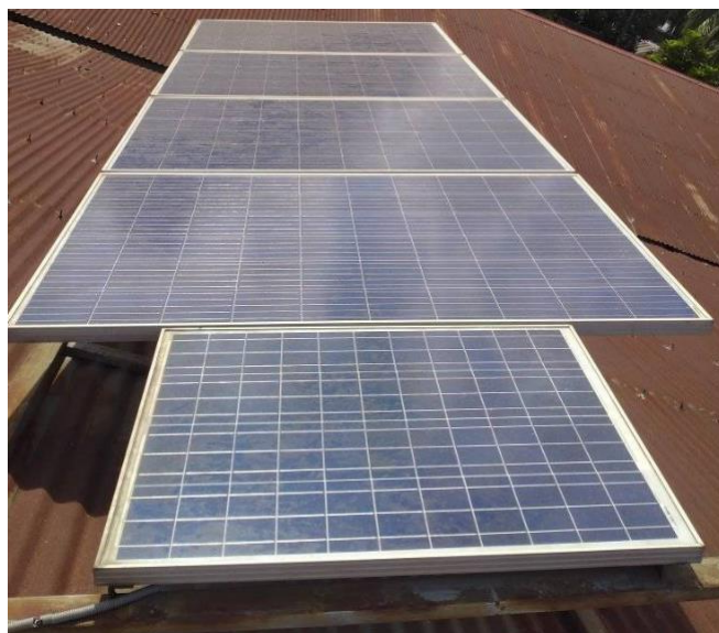
Figure 4.1: Solar system in Rooftop
