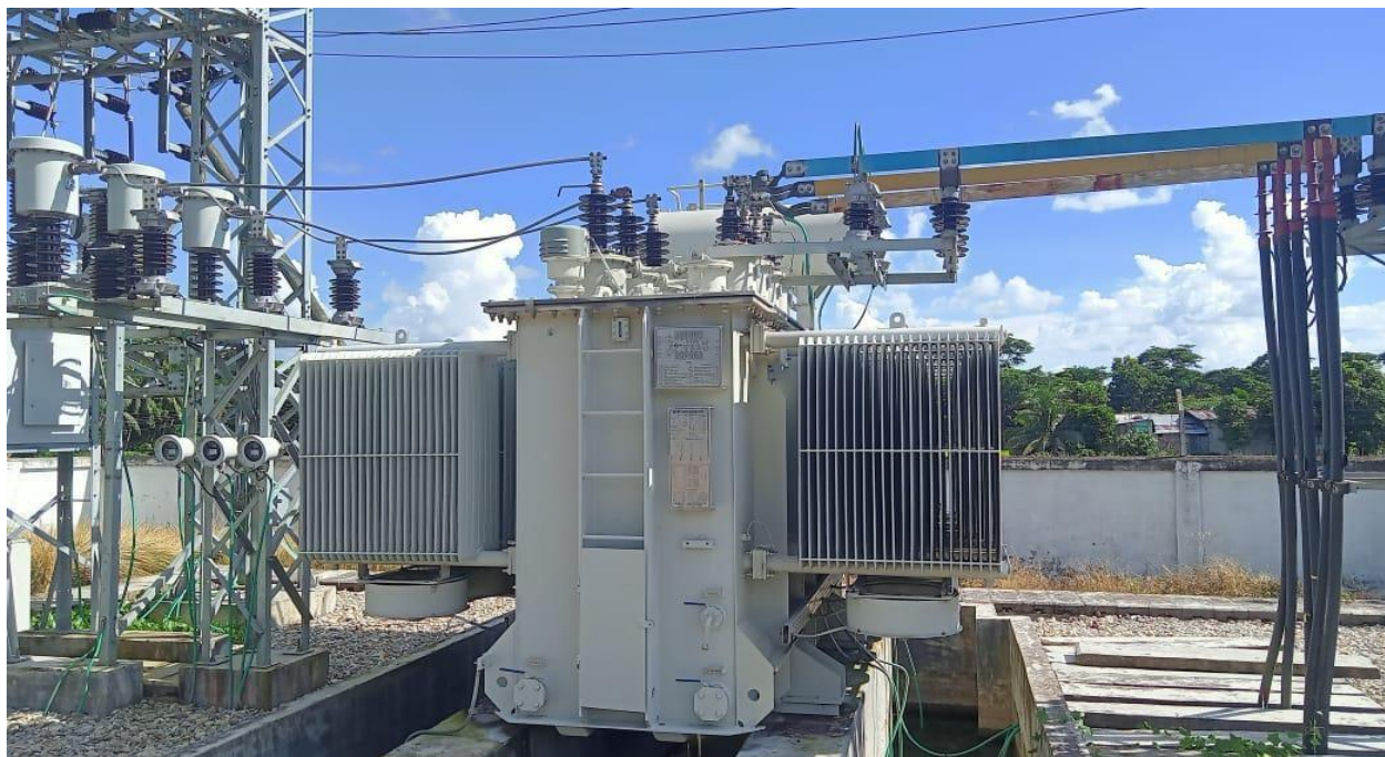
10/14MAV transformer (33/11 indoor substation, Maispara,Kalkini-2,MPBS)
