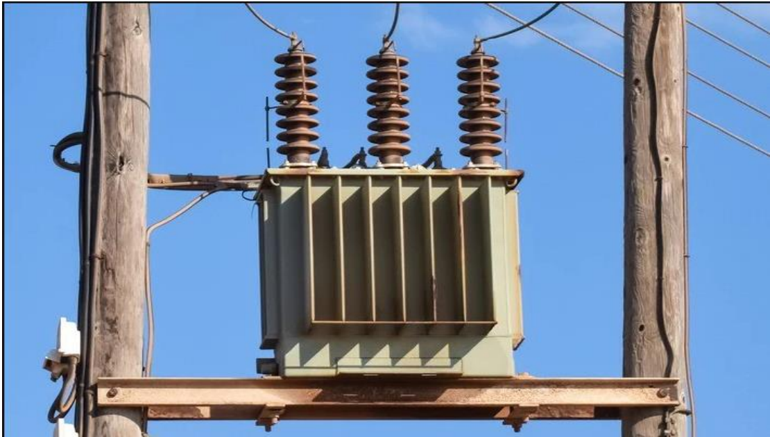
Figure1.1: A Distribution transformer
