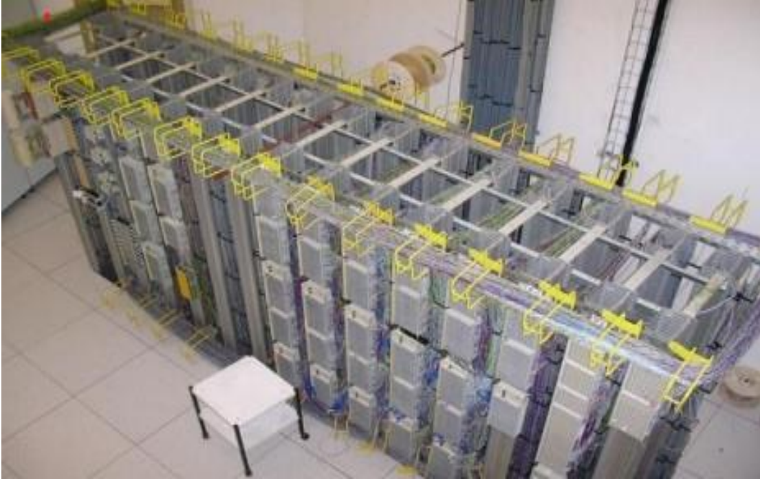
Fig: 5.4 Main Distribution Frame
