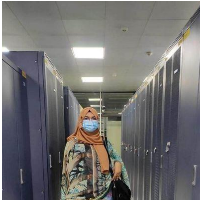
Figure: 6.1: Working time in switch room
