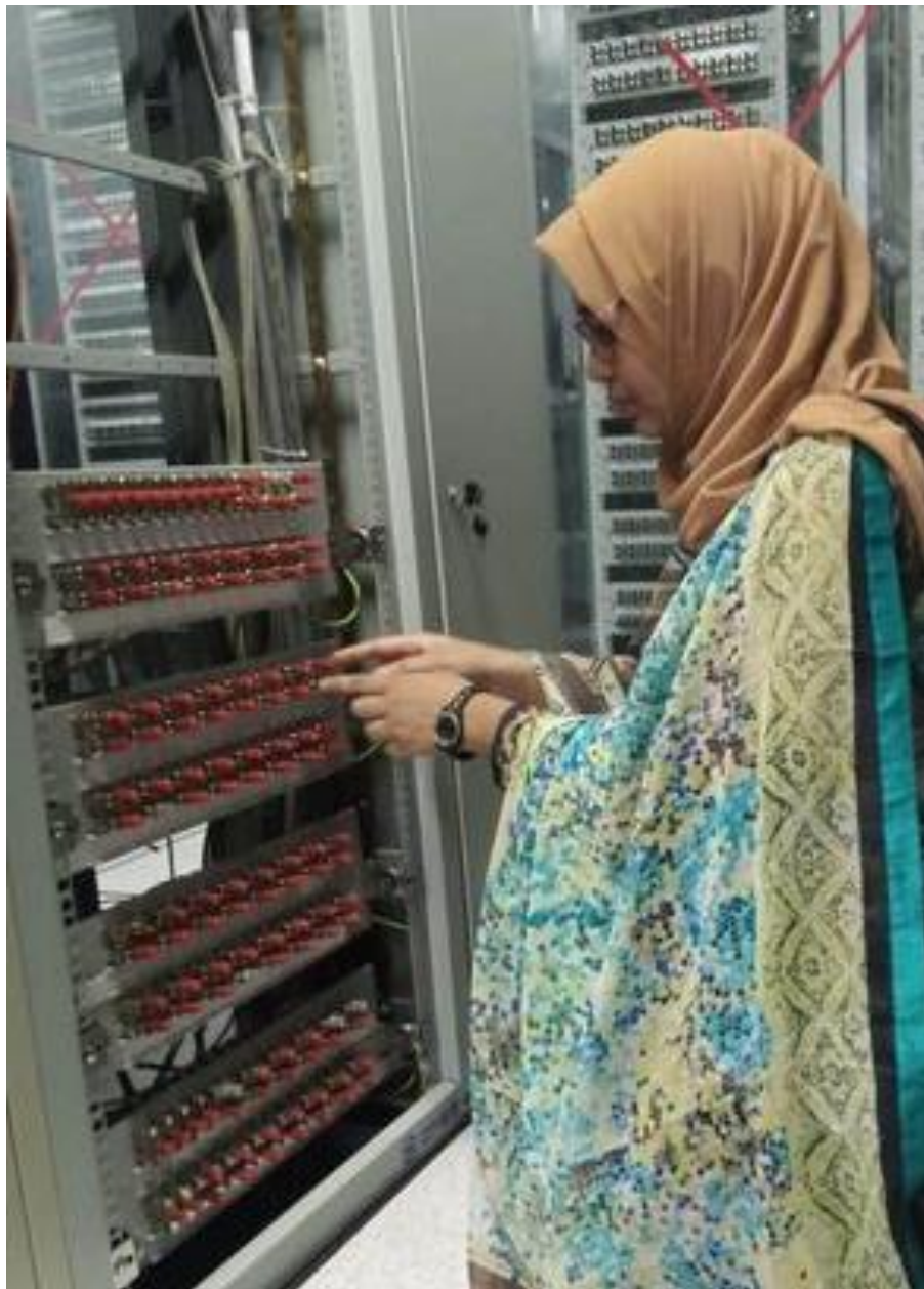
Figure: 3.3: Fundamentals of Out side plant & MDF
