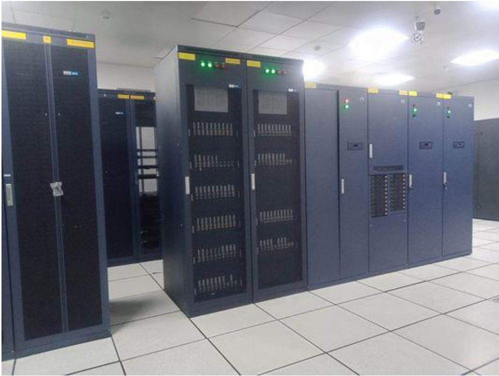
Figure: 6.2: Switch room
