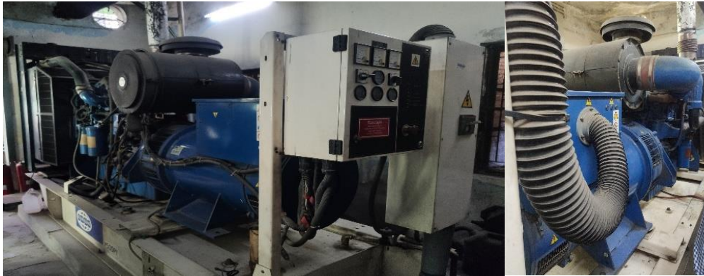
Figure 6.4: BTCL Generator Room
