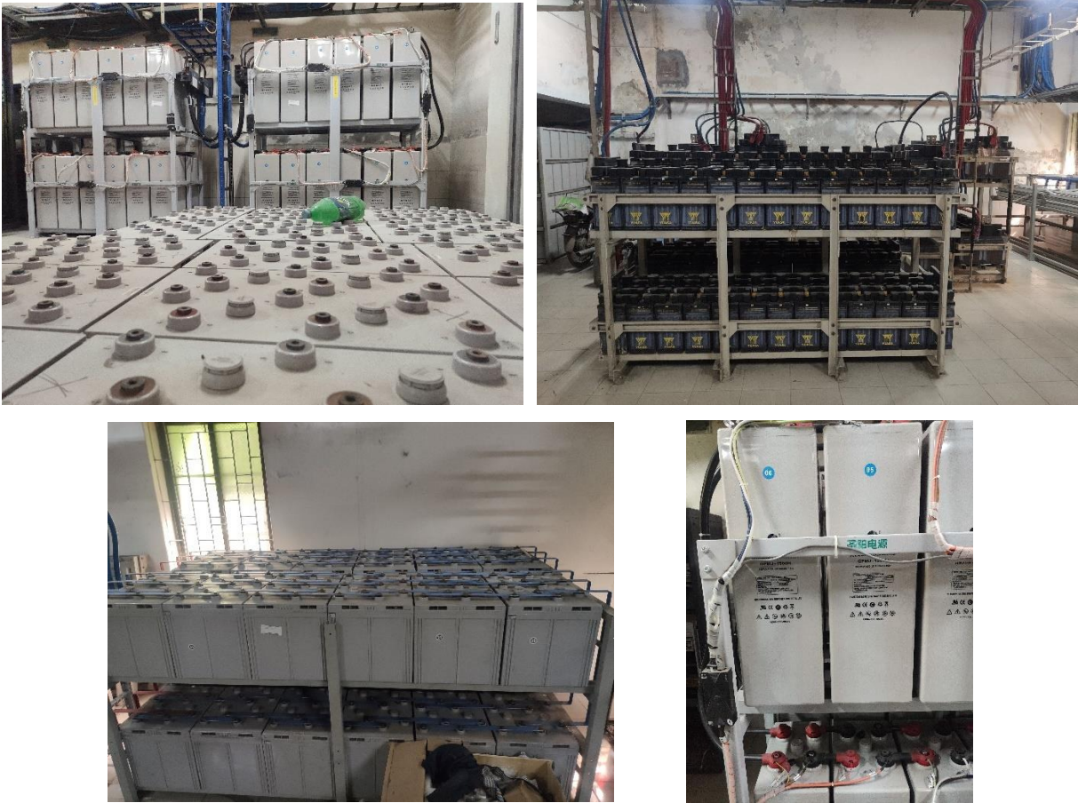
Figure 6.3: BTCL Battery Room
