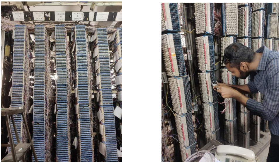
Figure 3.3: PSTN main distribution Switch room and Working
