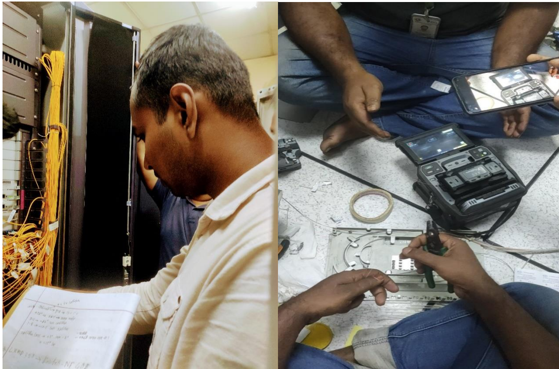
Figure 3.8: Fiber core connection and power measurement
