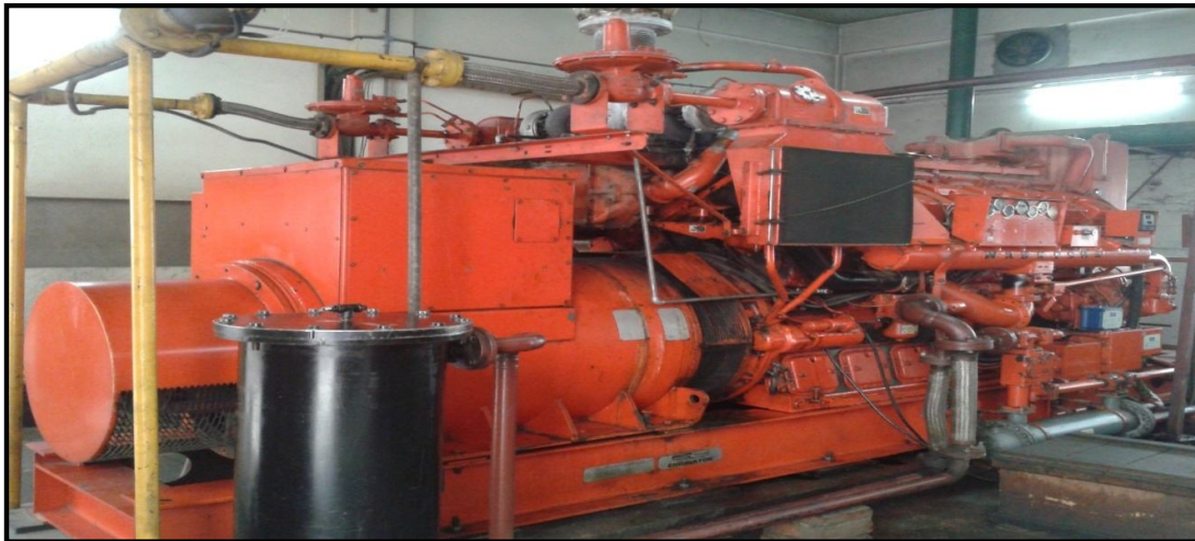
Waukesha gas Generator
