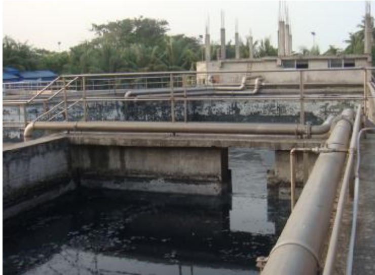
Figure-35: ETP Plant
