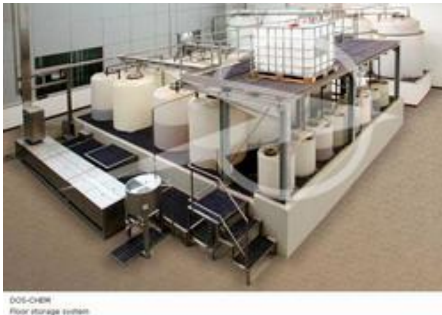
Figure-29: Chemical dosing storage tanks
