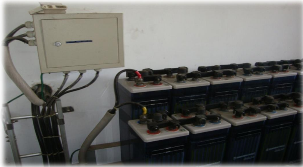
Fig 1.17: Storage Batteries. Image from[15]
