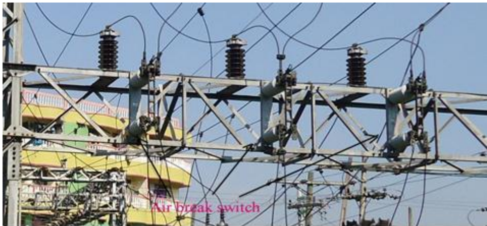
Fig 6.12: Air break switch
