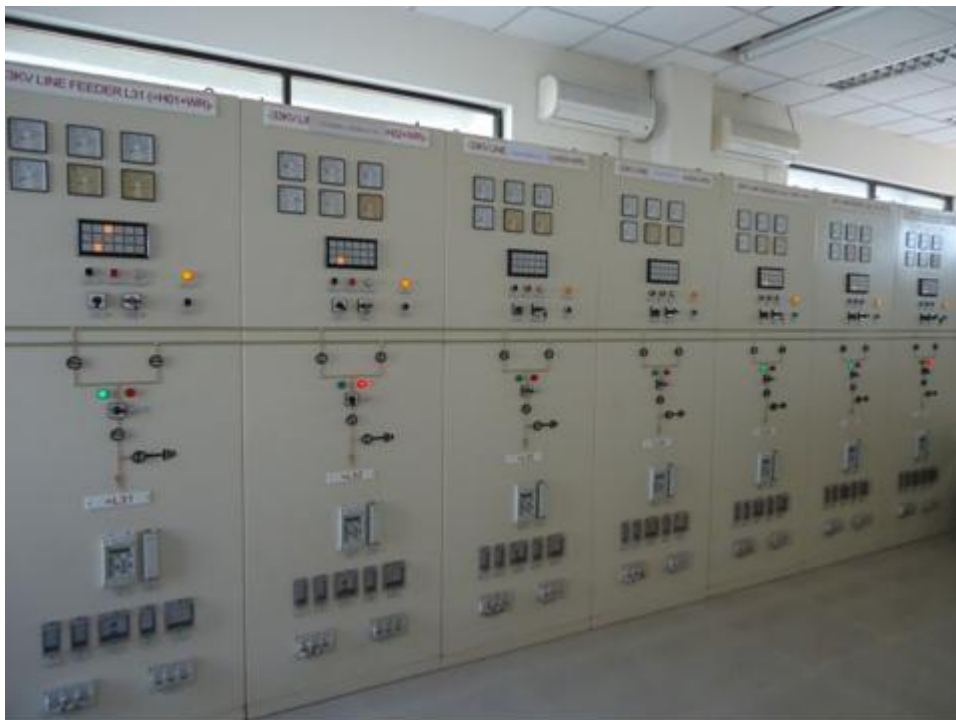
Fig 9.1: Control Room for 33KV Switching sub-station
