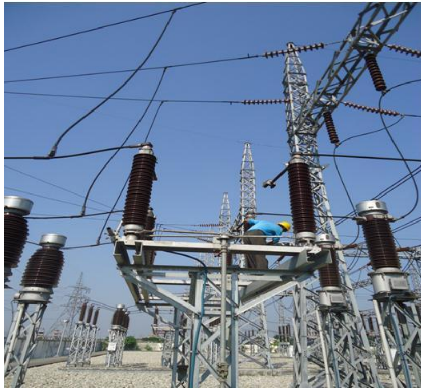
Fig 11.3: Fixed contact is taken out for to maintenance
