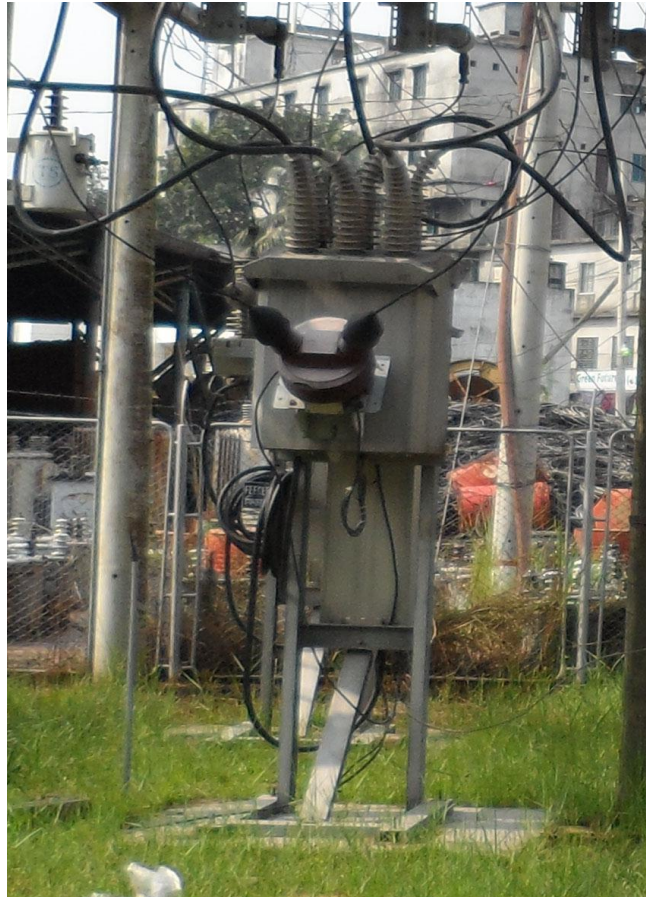
Fig 6.10: SF6 Circuit Breaker
