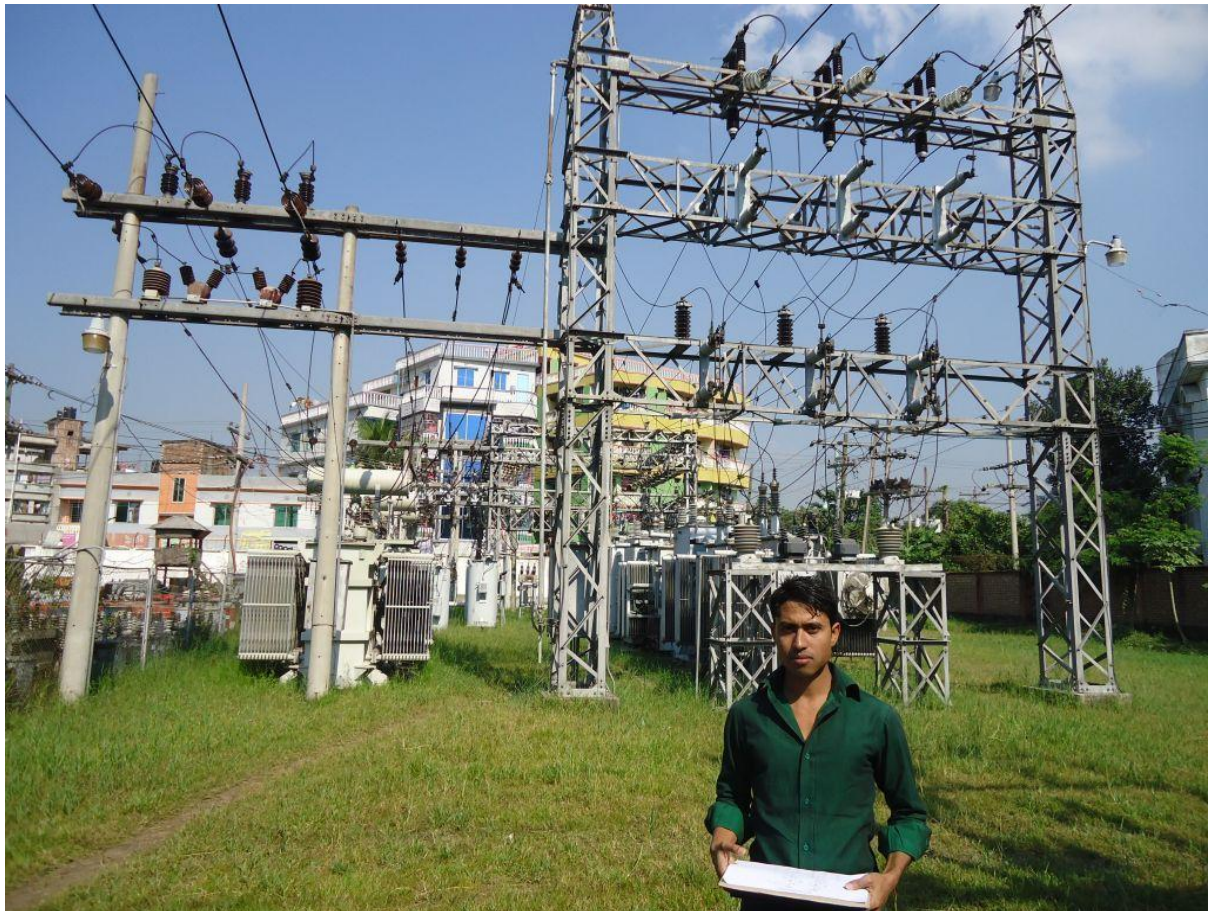
Fig: 5.1 33/11 KV Sub-Station ,DHAKA PALLI BIDYUT SAMITY-1,SAVAR
