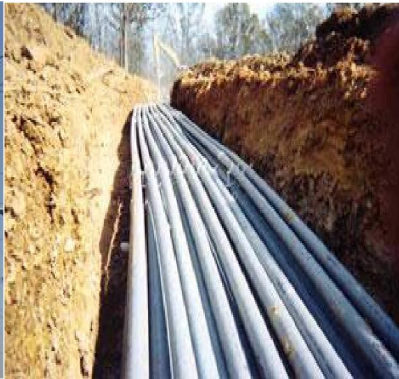
Fig: 3.3 Underground Transmission line
