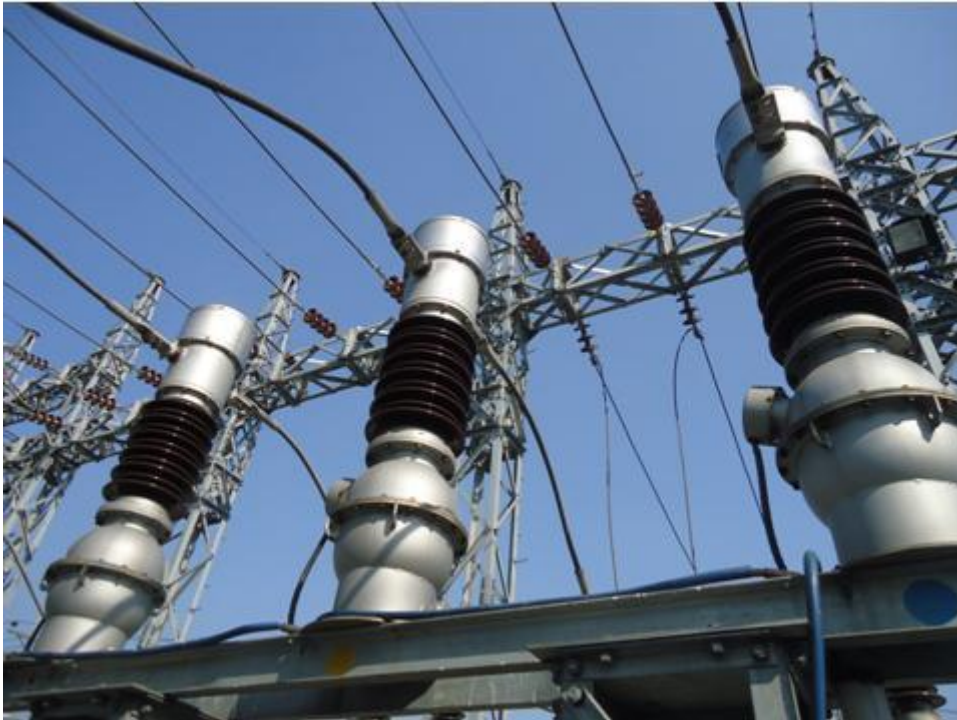
Fig 7.8: Current transformer CT
