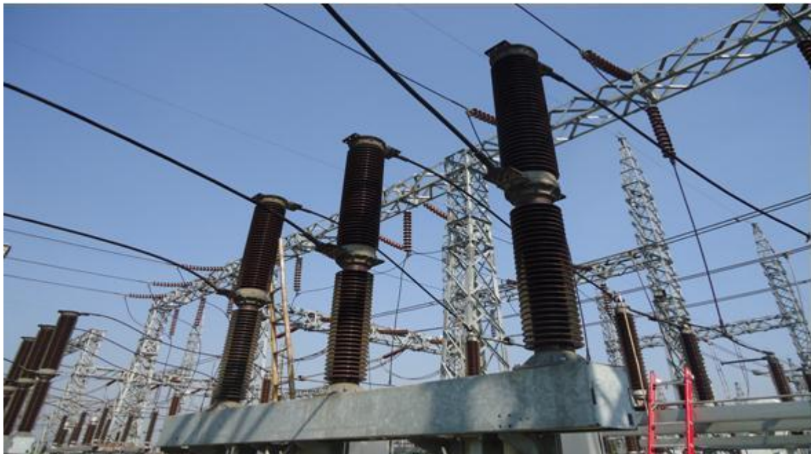
Fig 8.6 : Automatic Circuit Recloser
