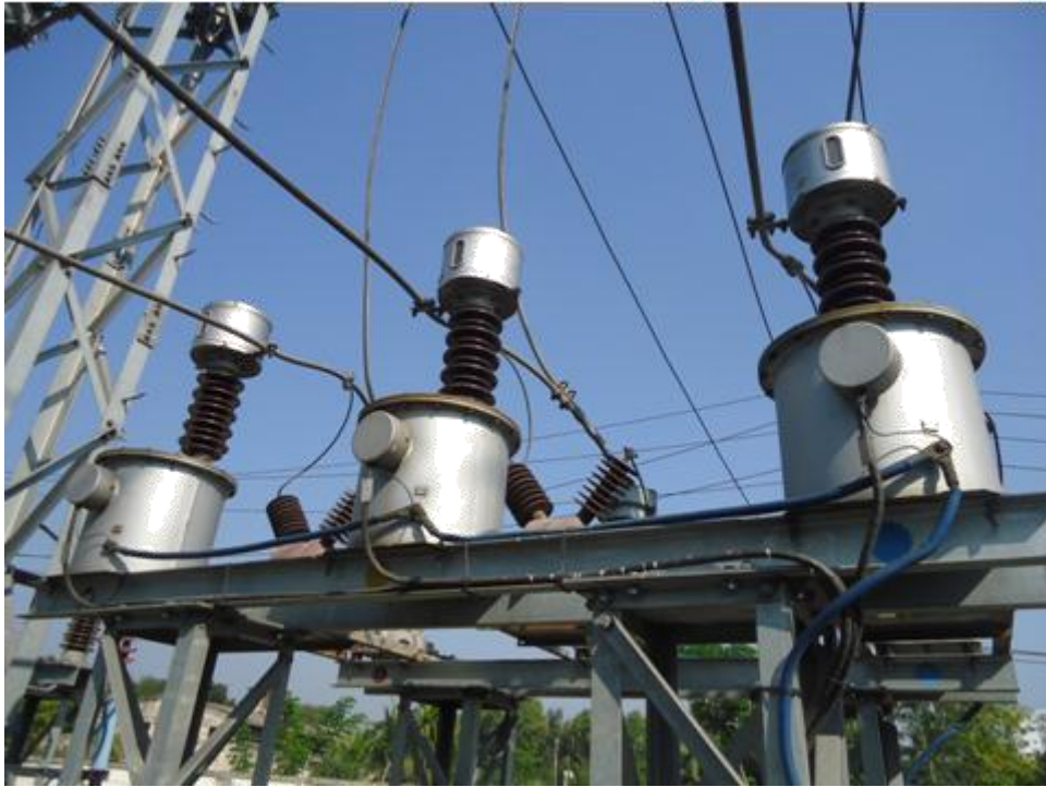
Fig 7.9: Potential Transformer PT
