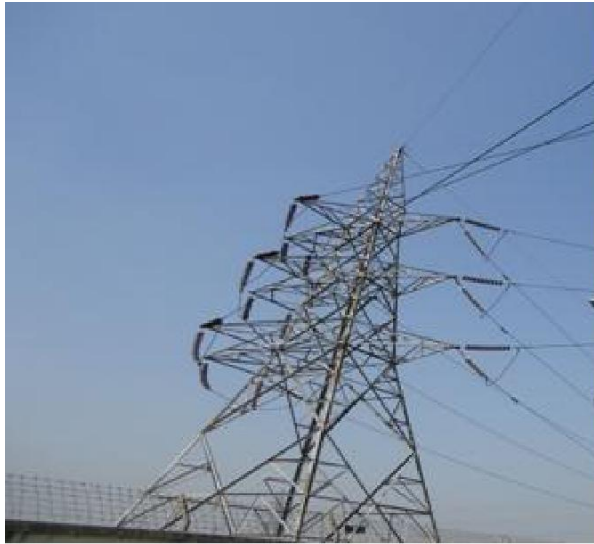
Fig: 3.2 Overhead Transmission line
