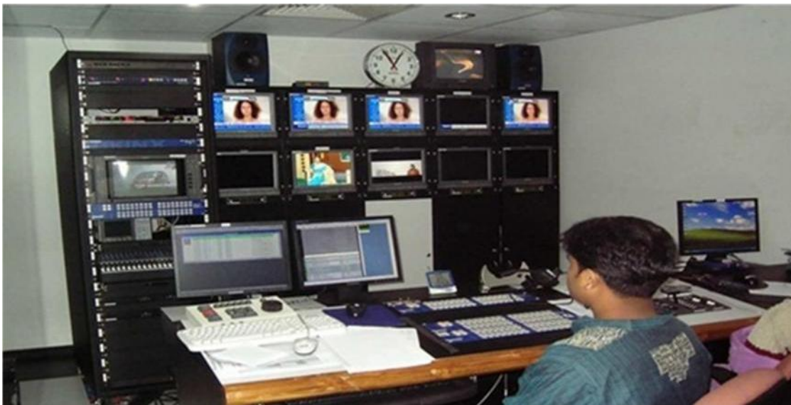
Figure 5.1 inside the Master Control Room (MCR)
