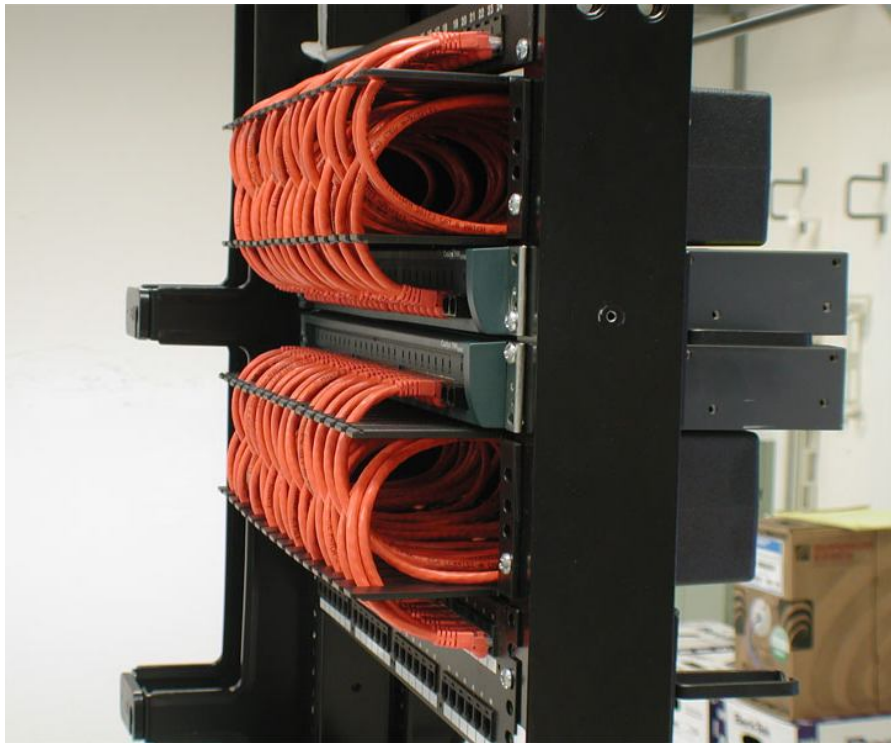
Figure 8.2: Managed Cable plug in Patch panel to Switch.
