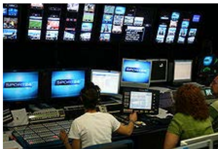
Figure 7.2: production control room (PCR)
