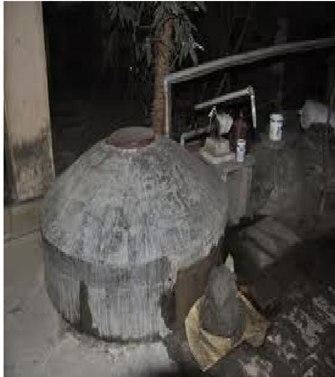
Figure14: An under constructed Bio-Gas plant and complete Bio-Gas Plant investment by EXIM Bank.
