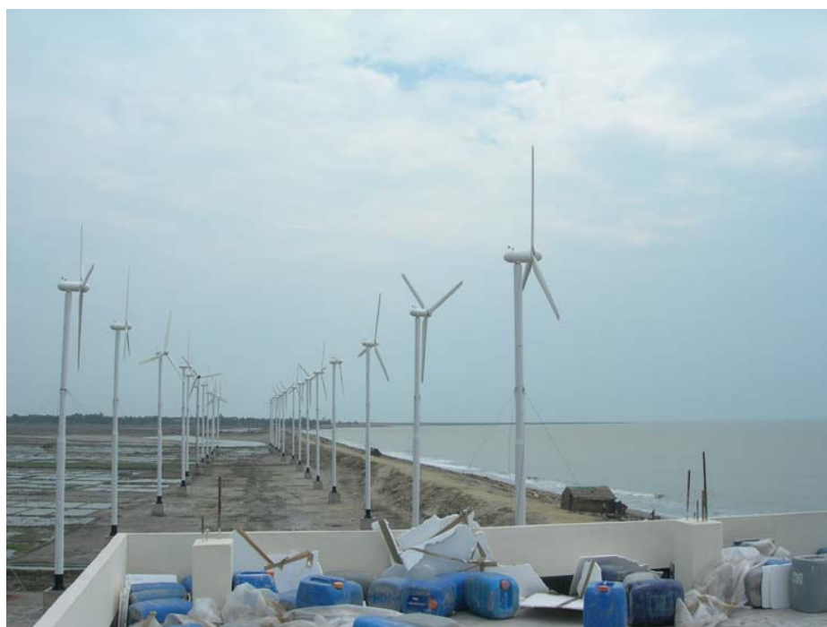
Fig:8.3 1000 Kwp capacity wind battery hybrid system power plant of Kutubdia
