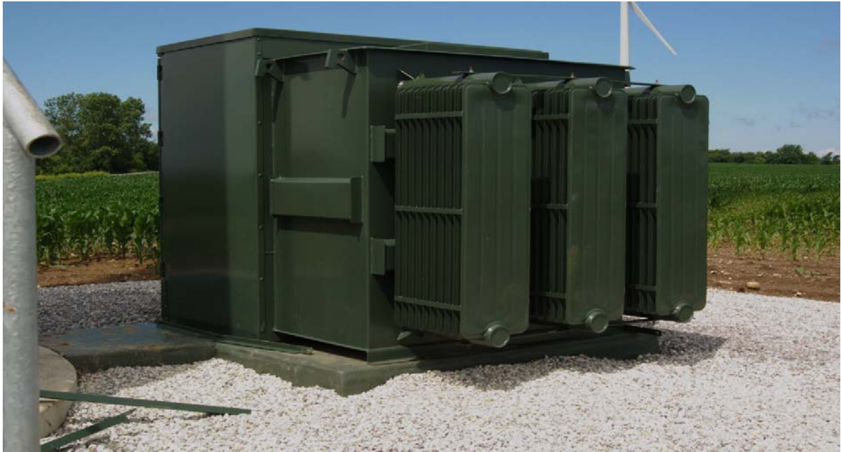
Fig: 3.2 Transformer of wind turbine
