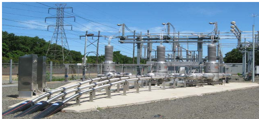
Fig:6.2 Transmission line of electricity
