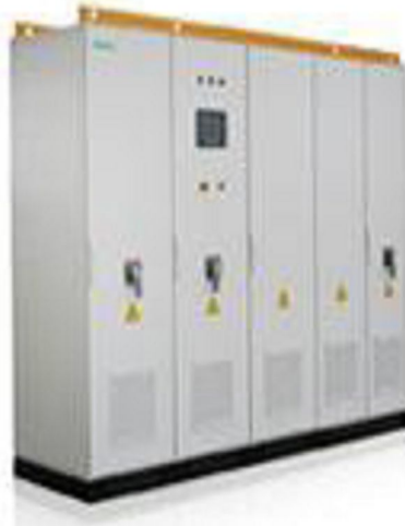
Figure2.20: Power plant inverter
