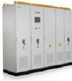
Fig20:Power plant inverter
