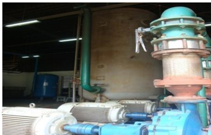
Fig: Water supply pump
