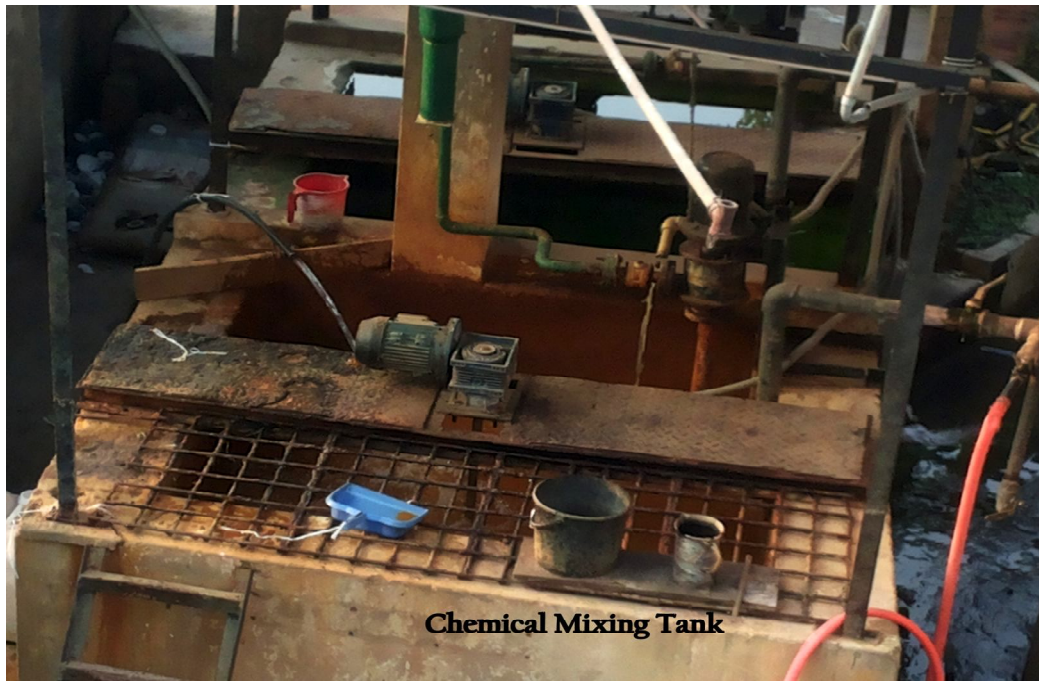
Figure 4.6: Chemical Mixing Tank
