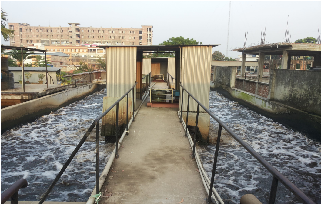
Figure 4.5: Pictorial View of ETP at DTL
