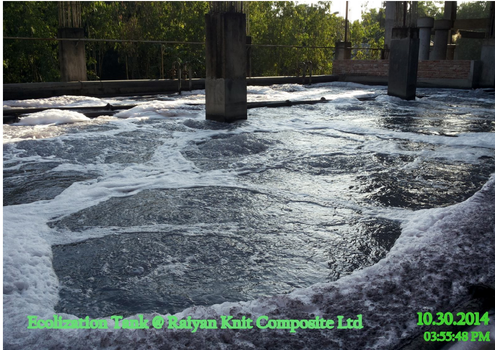
Figure 4.16: Ecolization Tank at RKCL
