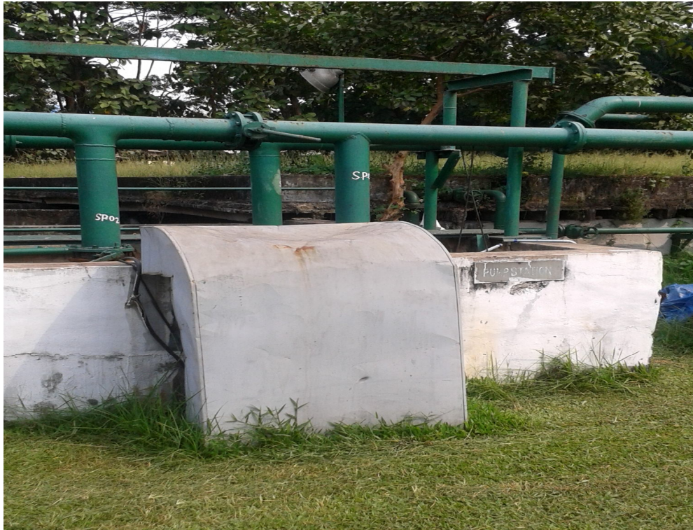
Figure 4.14: Pump Station of ETP at BTL
