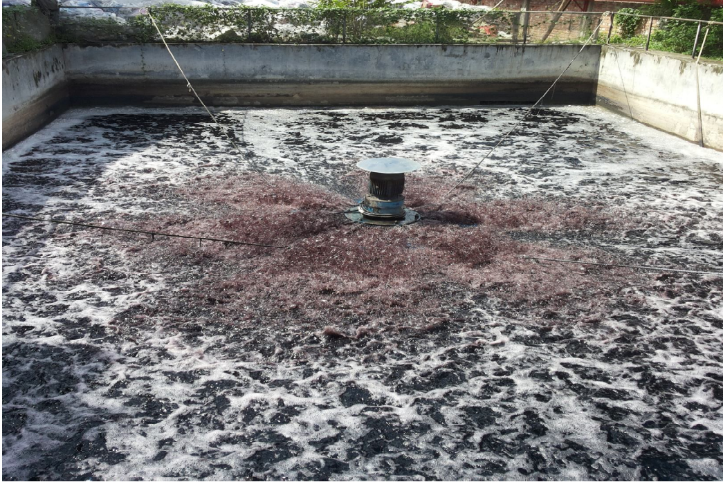
Figure 4.4: Pictorial View of ETP at DTL
