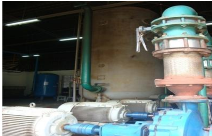
Fig: Water supply pump
