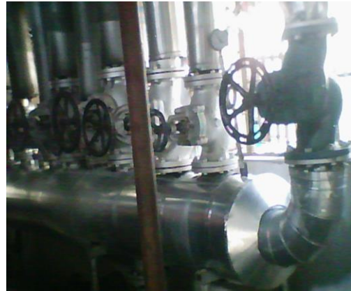
Fig: Steam Delivery Chamber
