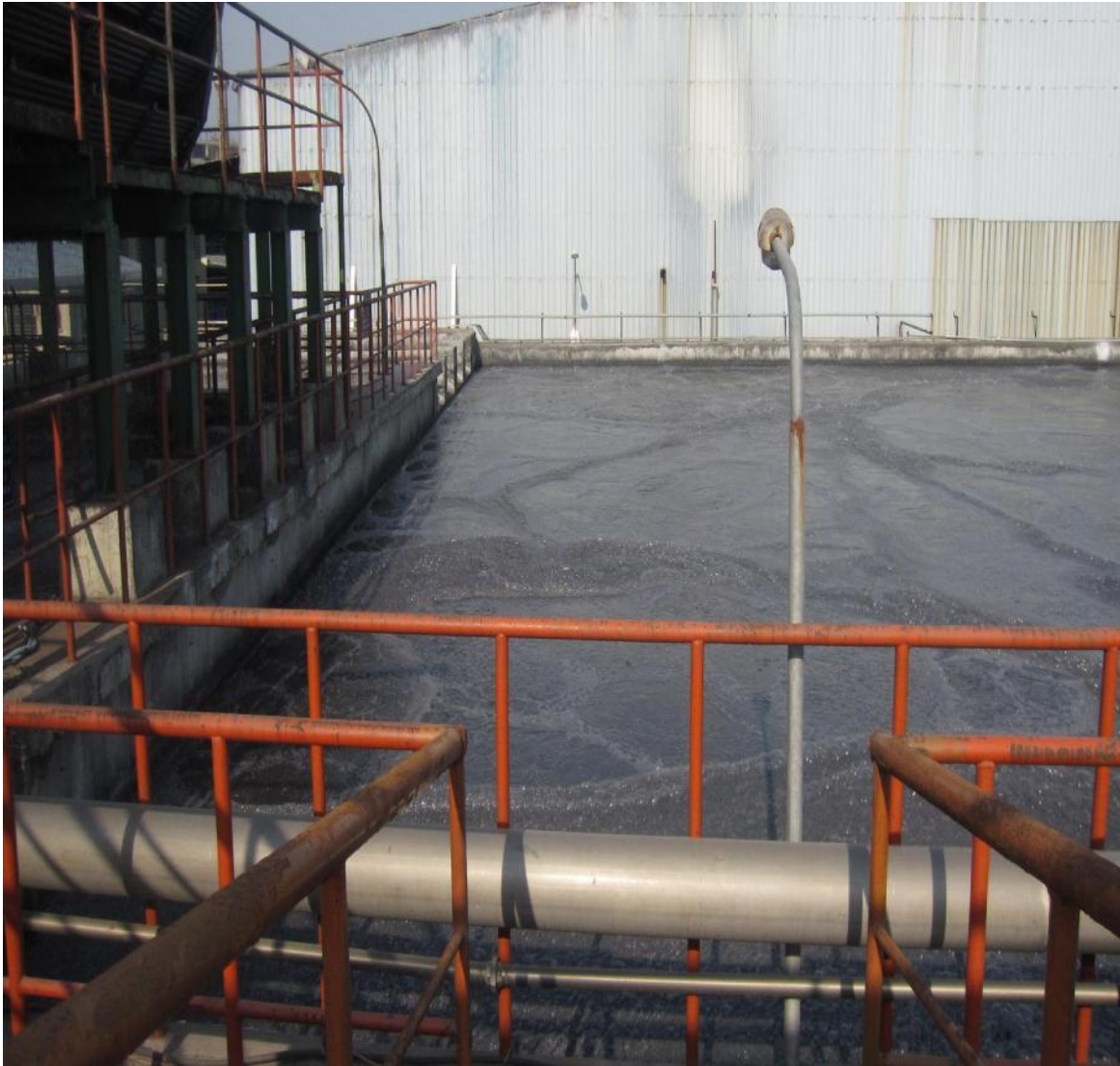
Figure: Effluent Treatment Plant
