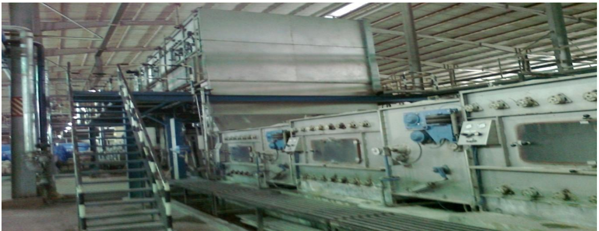
Fig: Scouring and Bleaching M/C
