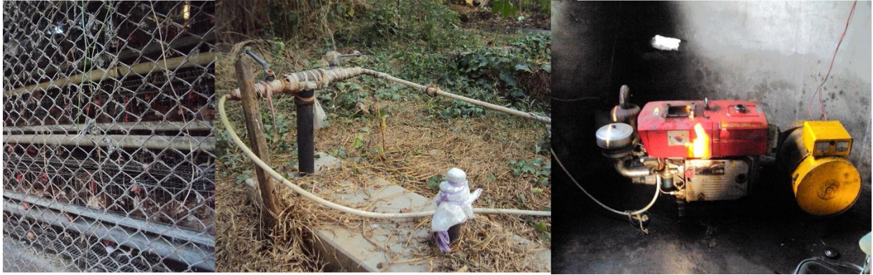
Fig:16 Picture of 10 kw biogas power plant in Bahuria chala, Bhawal Mirzapur, Gazipur-1703
