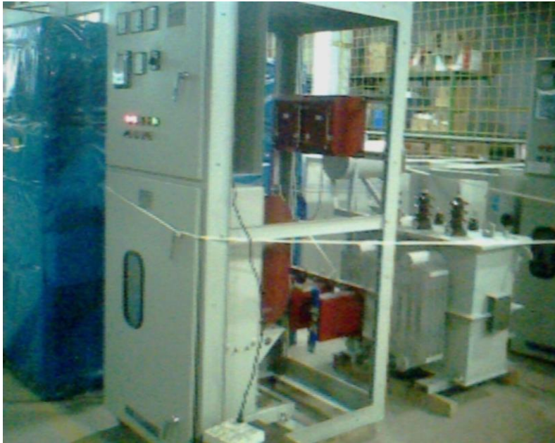
Figure 25: BSC equipment room
