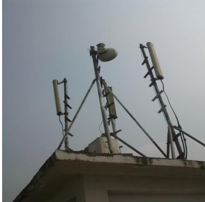
Figure 33: GSM microwave antenna
