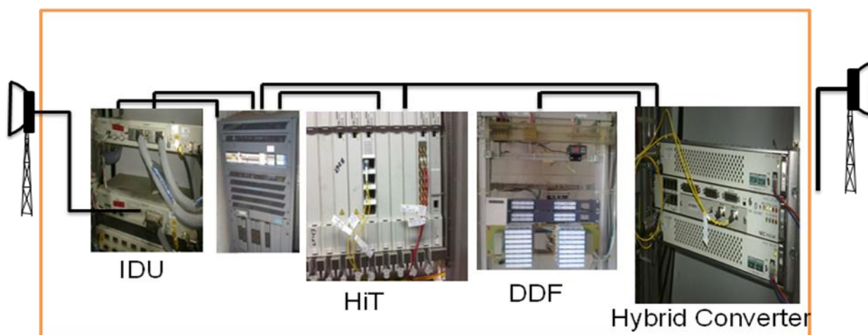
Figure(3.4): HiT Room
