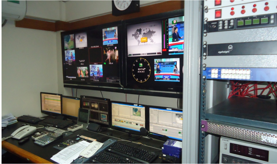
Figure 12.1 inside the Master Control Room (MCR)
