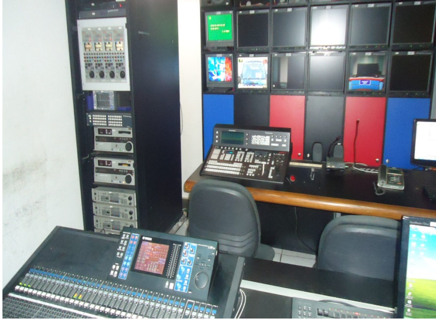
Figure 6.2 inside the Production Control Room (PCR)[1]
