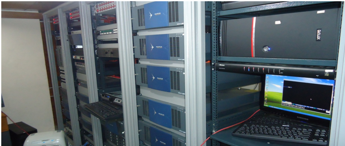
Figure:11.1 Central Apparatus Rooms
