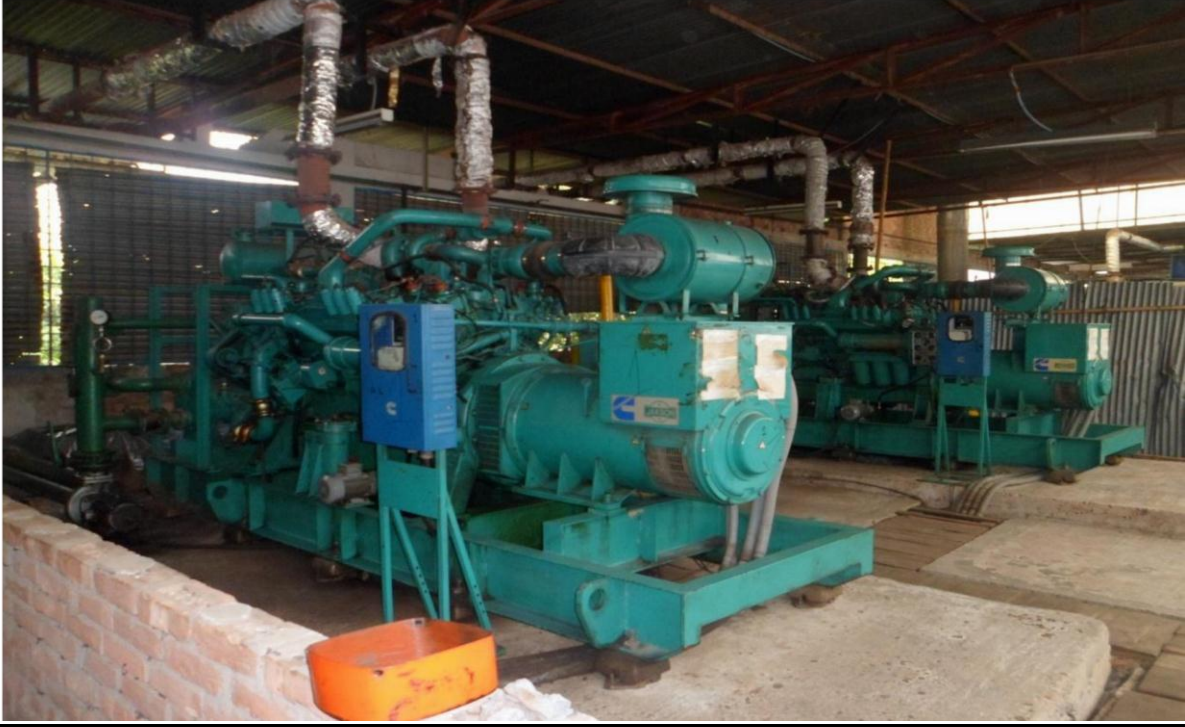
Figure: Gas Generator
