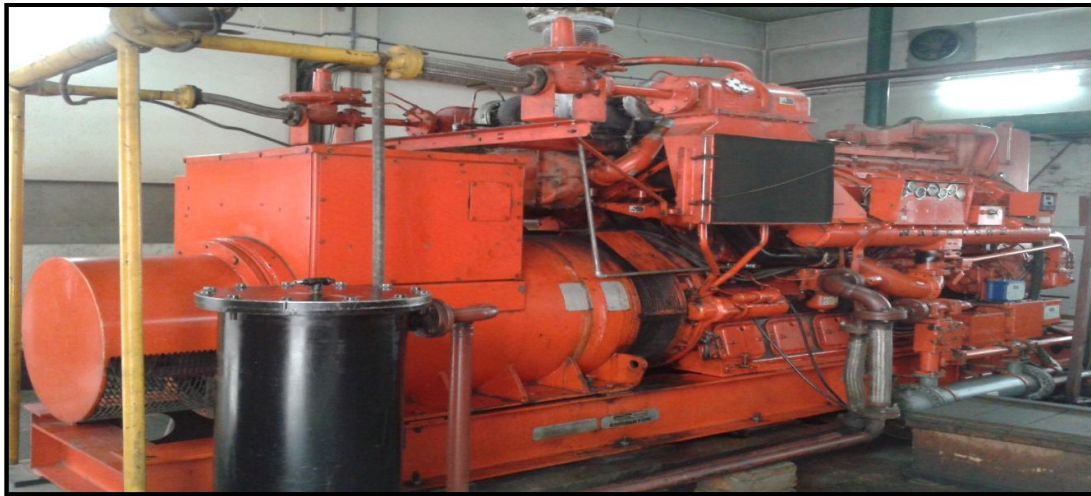
Waukesha gas Generator
